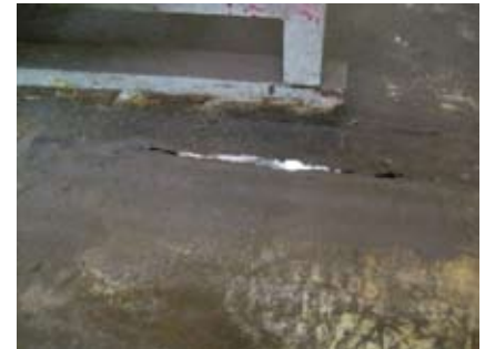
Picture7: case V Cracking on the top of tank
