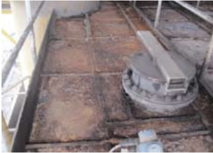
Picture3: case III Corrosion on top of tank
