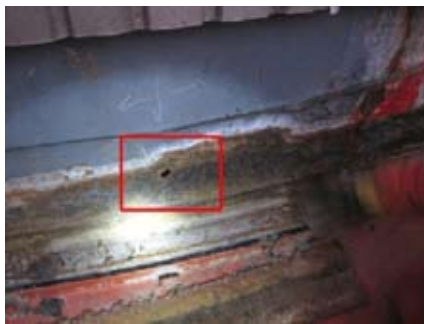
Picture1 : case I Leaking point
