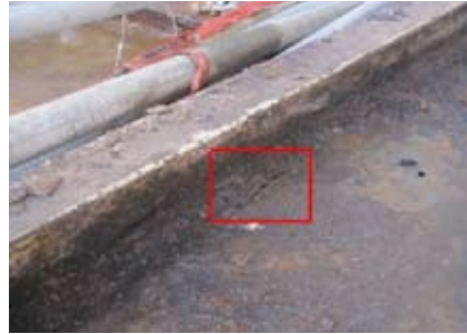
Picture4: case III Cracking on the top of tank
