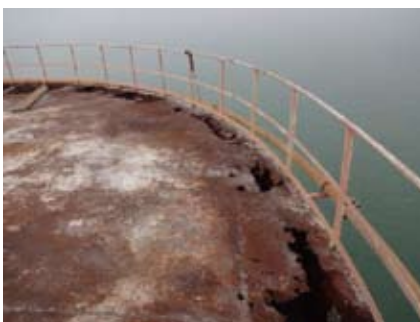
Picture5: case IV Corrosion on top of tank
