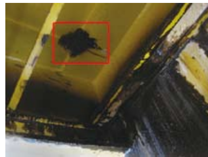
Picture2: case II Leaking point
