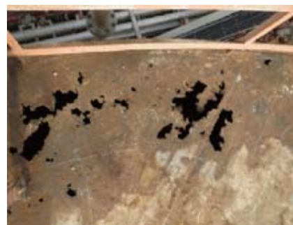
Picture6: case IV Corrosion on top of tank
