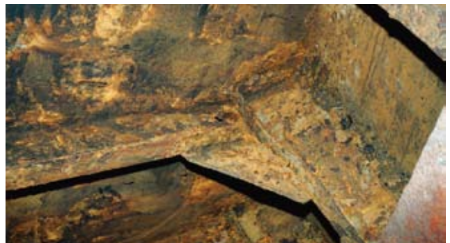
Figure 1 The serious corrosion at the top of aging oil tank
