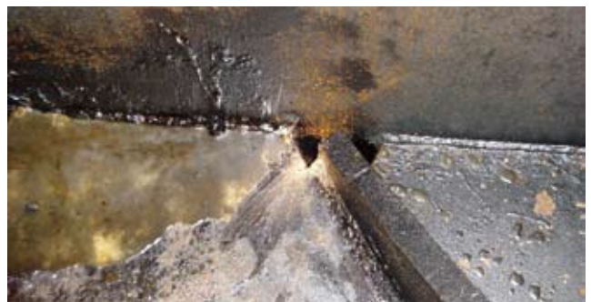
Figure 2 Pitting corrosion at the bottom of oil hold of two-year-old tanker
