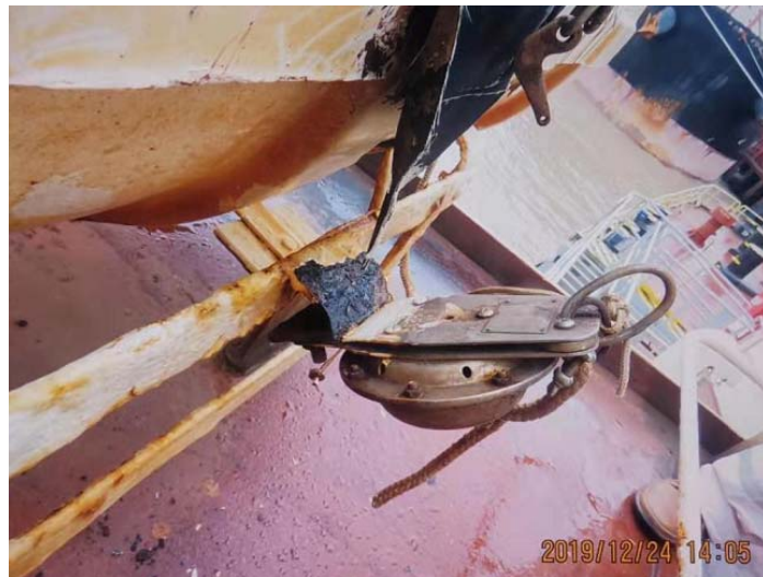
Foundation of HRU serious corroded
