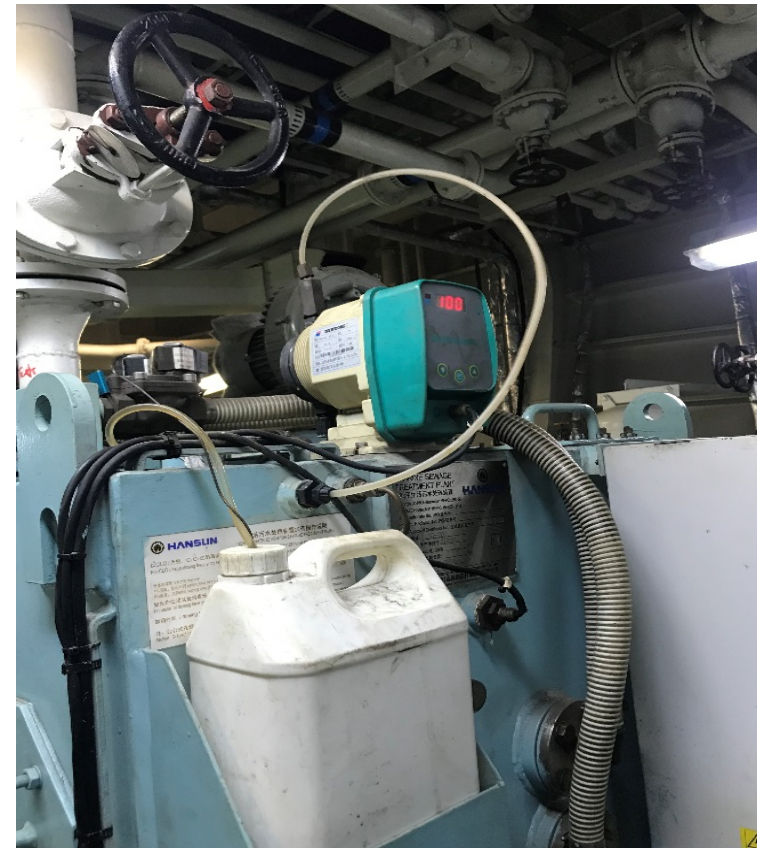
Disinfectant pump for sewage treatment plant inoperative
