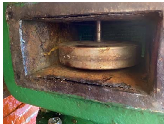
Air vents and closing arrangements defective
