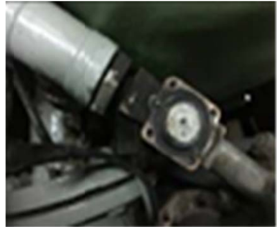
Engine room bilge pump is inoperative
