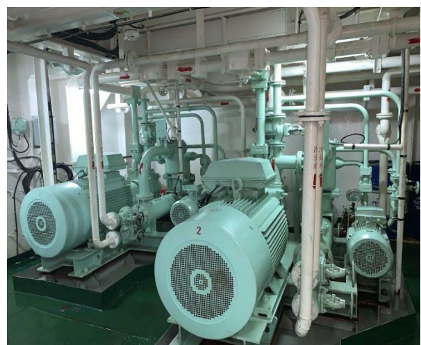
Hydraulic oil on electric box of pump motor
