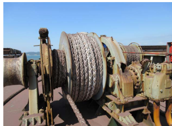
Mooring rope poor condition
