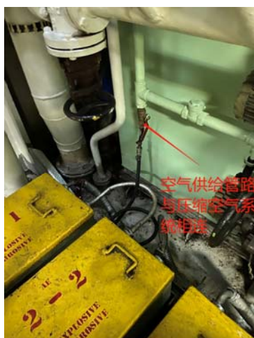
Sewage treatment plant defective (air pump not work)
