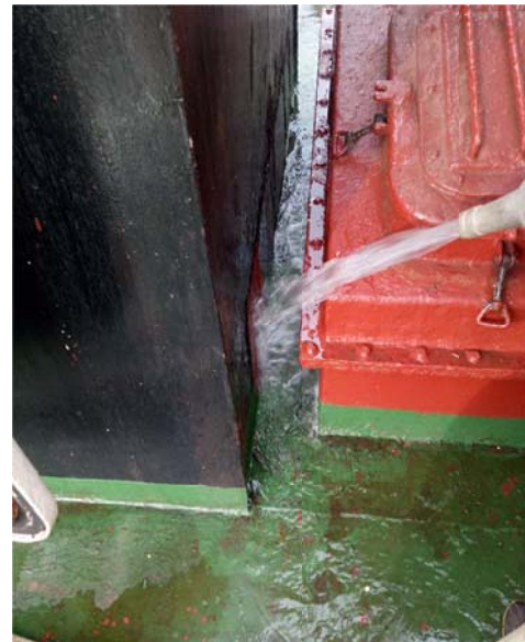
Funnel fore BHD—corroded and holed( repaired)
