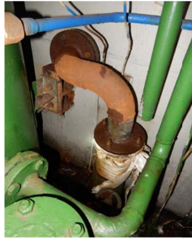
E/R E.F.P suction pipe with flanges
