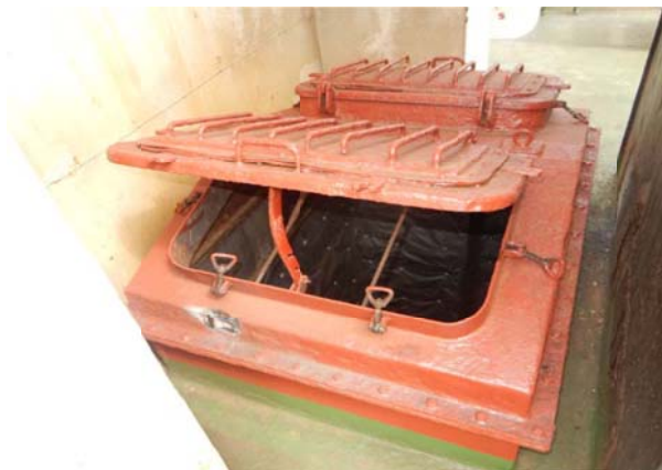
E/R skylight coaming corroded and holed
