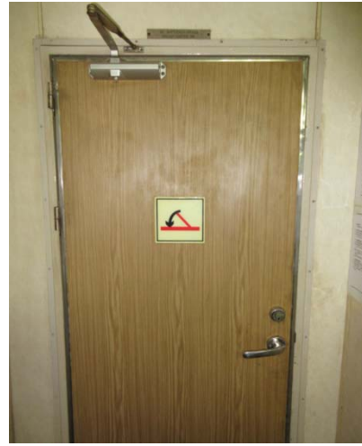
Fire door self-closing device-defective
