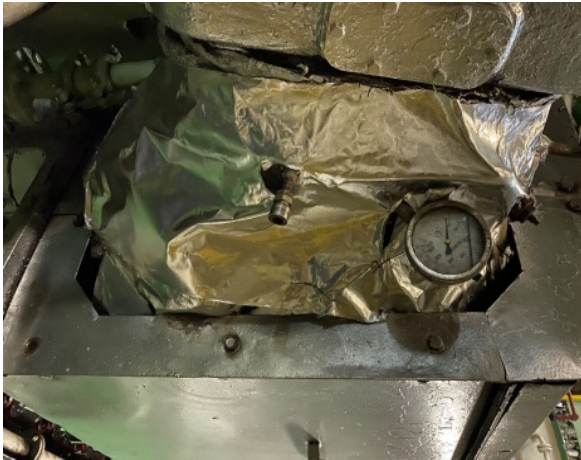
Heat insulation lagging missing (rectified)
