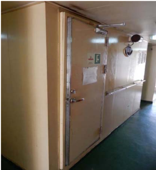
Fire door self-closing device damaged.
