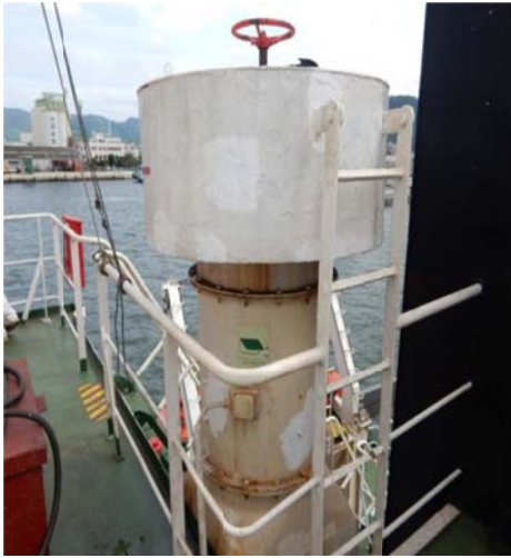
Fire damper of E/R vent—unable to close smoothly
