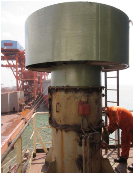
Engine Room fire damper defective
