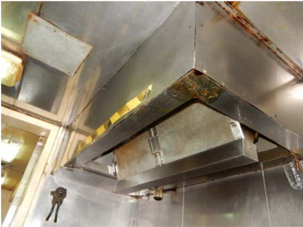
Galley duct for ventilator—dirty with oil
