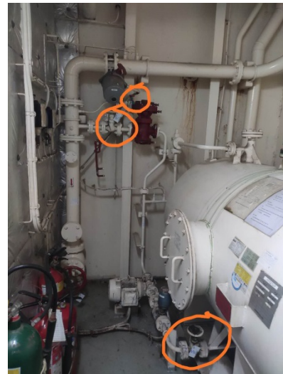
Foam fixed fire extinguishing system three operating valves closed (opened normally)
