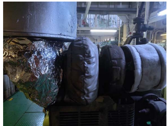
Turbo charger and exhaust trunk insulation defective
