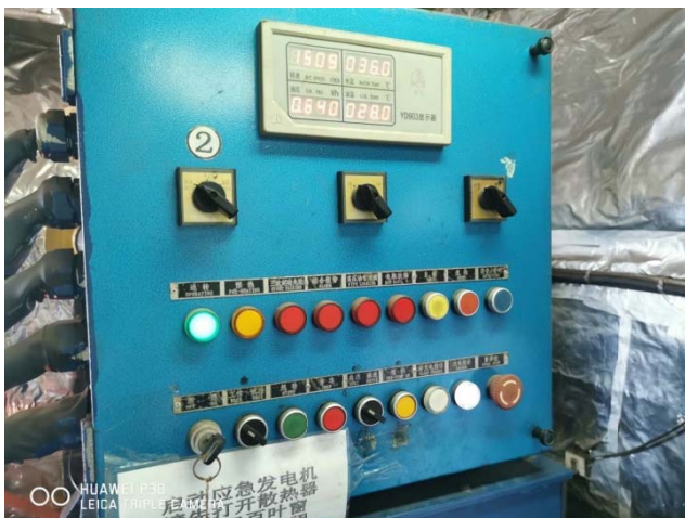
Emergency Generator found defective
