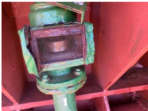
Air vents and closing arrangements defective
