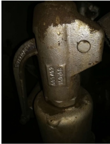
Lever pin of boiler safety valve removed, hand operation impossible.
