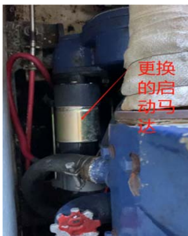
Life boat engine defective ( Starting motor renewed)
