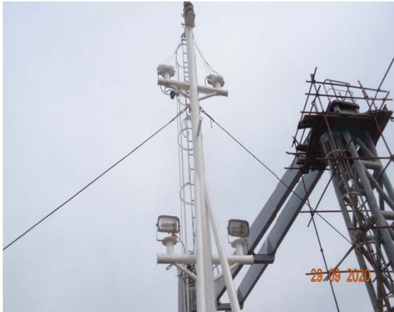
Forward mast stay wires defective (renewed)
