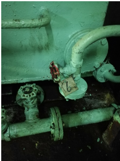
Sewage treatment plant scour air valve #(6) was opened (to be closed normally)
