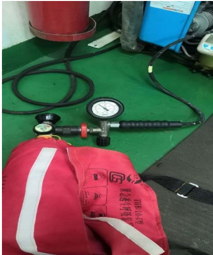
One EEBD in wheelhouse with insufficient pressure
