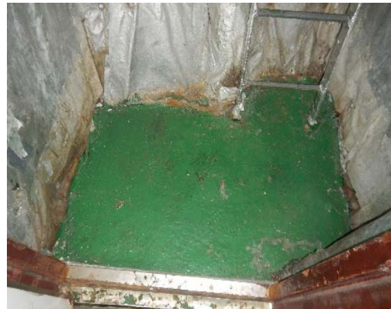
Escape tunnel bottom insulation damaged.
