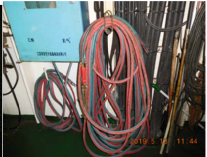
Oxygen and acetylene pipe aged
