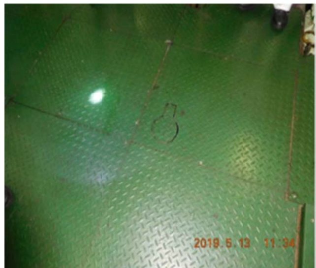
Engine room floor plates not fixed
