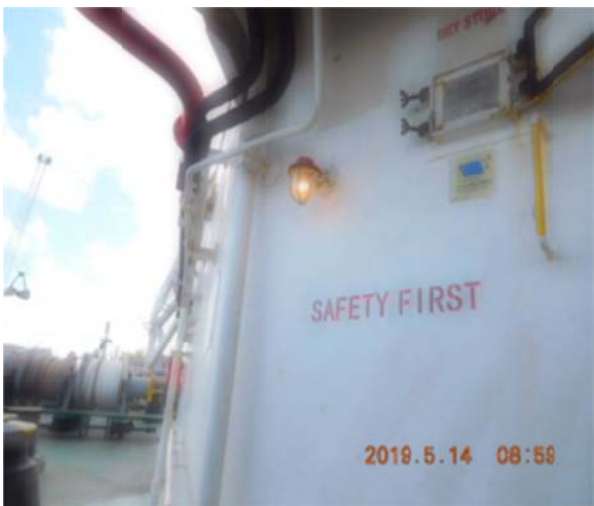
Emergency light unlit (rectified)
