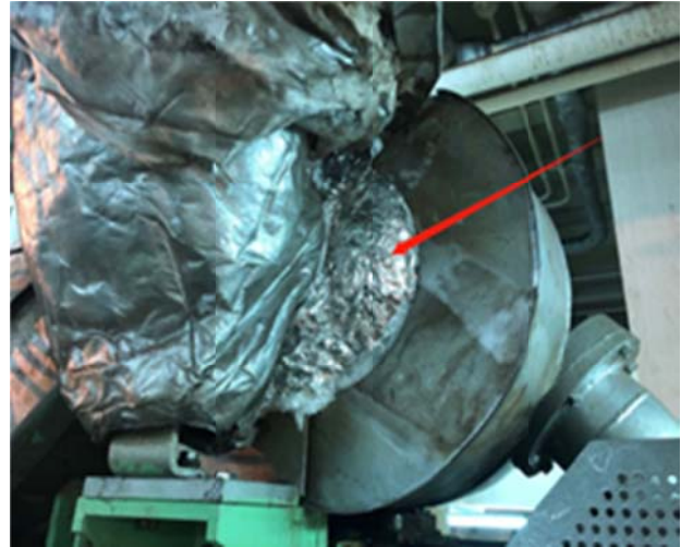
Turbocharger insulation damaged
