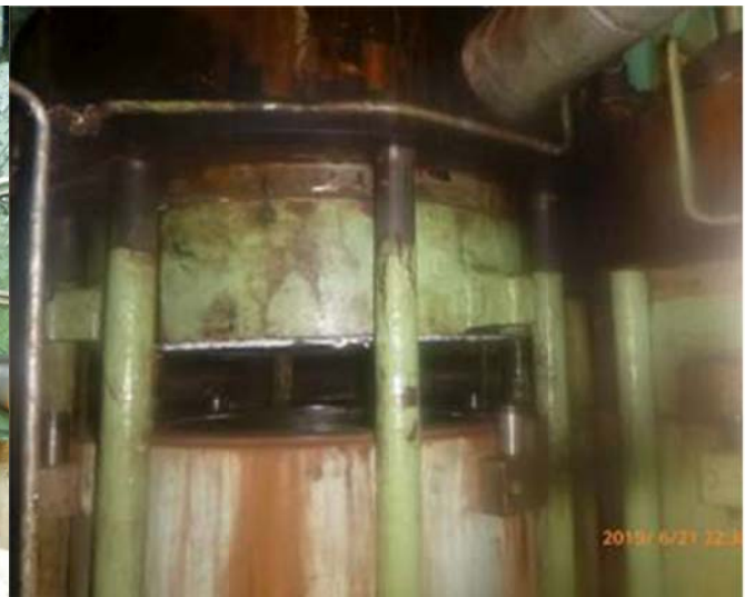
Main engine cylinder leaking water
