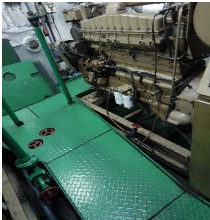
Unapproved cable and fan in engine room
