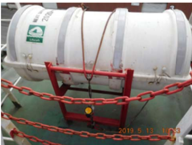
Life-raft cable not properly connected
