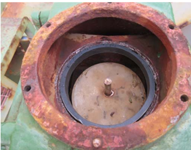
Rubber ring in ballast tank air pipe head damaged
