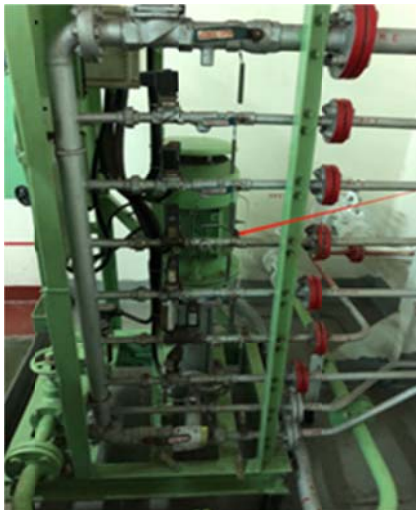
Water mist fire-fighting system not ready for use
