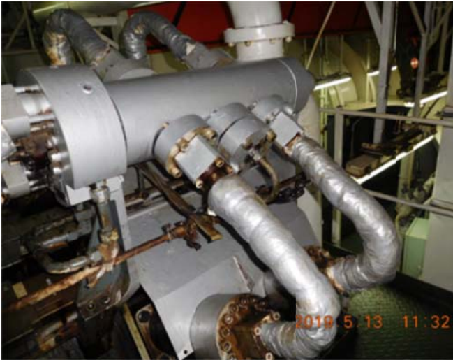
Main engine fuel oil leakage
