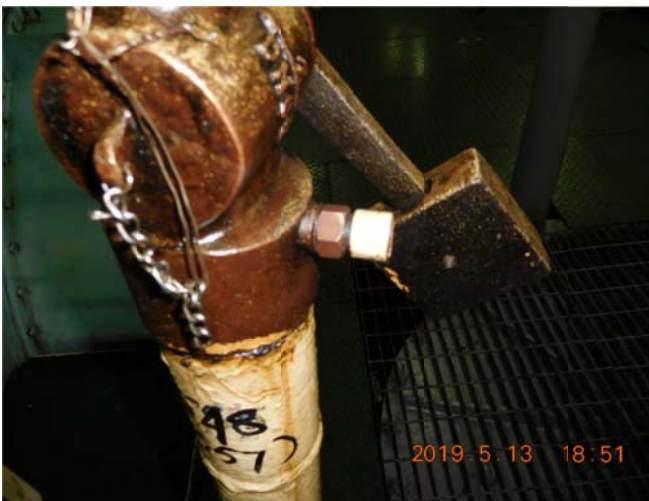
Oil tank self-close valve fixed in open condition (rectified))
