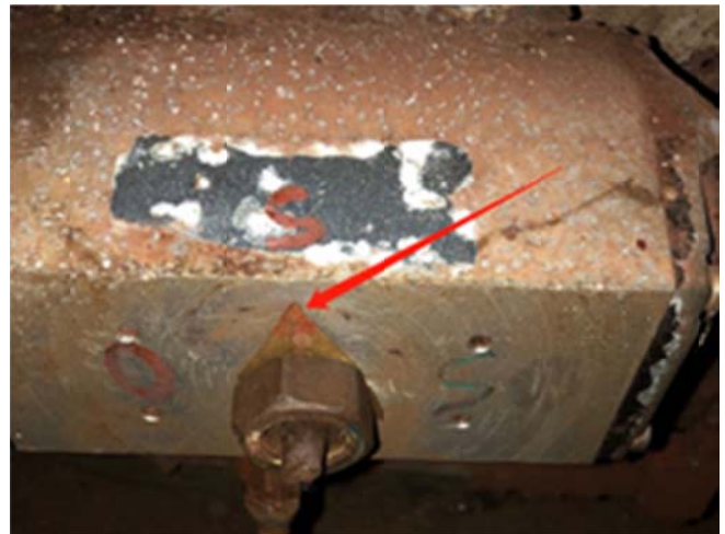
E/R ventilator damper direction missing
