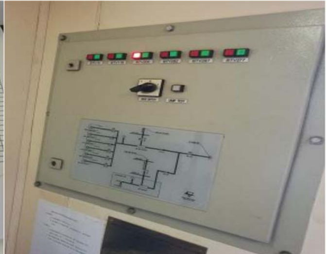
Bow bilge water remote control valve malfunction
