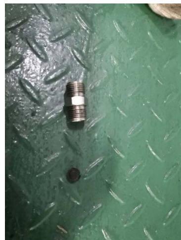
OWS sample pipe blocked by rubber ball
