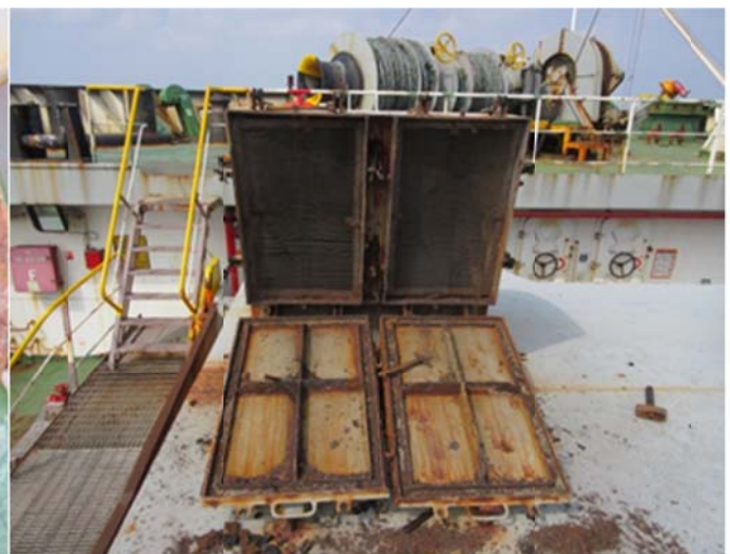
Rubber seal of cargo hold ventilator cover aged
