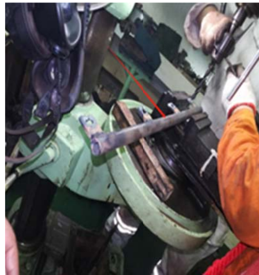
E/R ventilator damper could not closed totally
