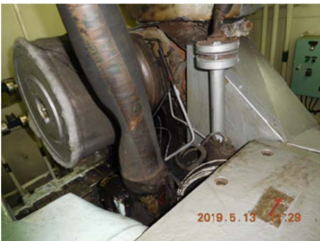
Detection of A/E turbocharger speed defective
