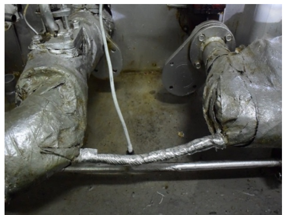
Isolation packages of high temperature pipes damage
