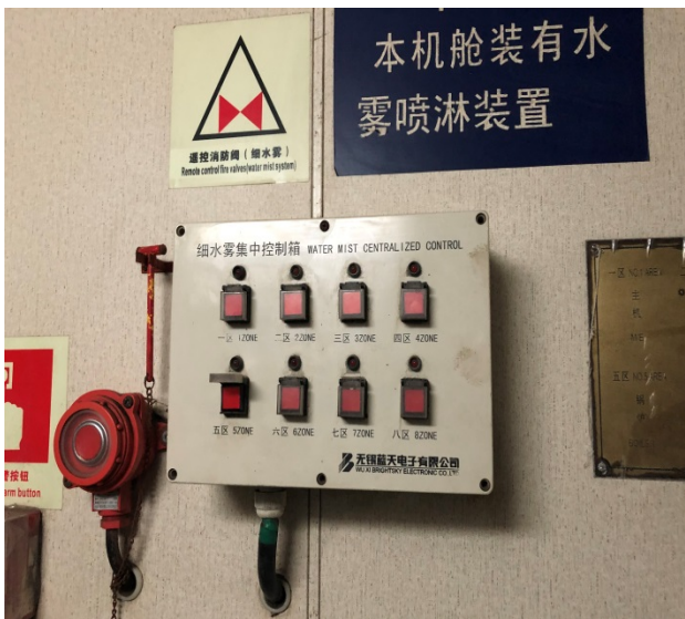
Fixed local application fire extinguishing system failure
