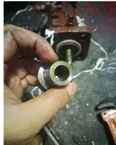
Emergency Generator oil tank quick closing valve defective
