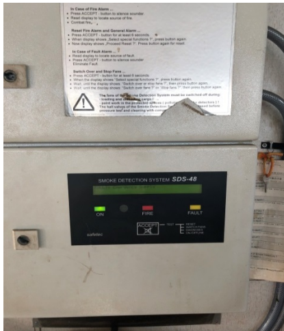
Cargo holds smoking detecting system failure
