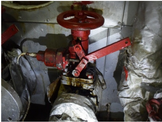
Oil tank quick closing valve defective
