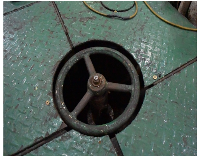
E.R. floor plates were not be fixed
