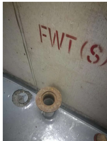
Cover of F.W. tank sounding pipe missing
