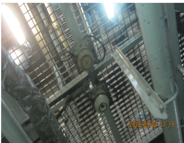
Fire detector failure
