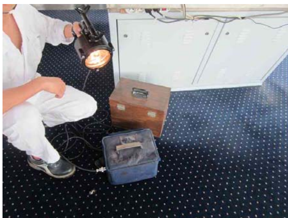
Portable battery of daily search light missing
