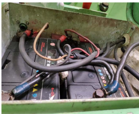
Starting battery of life boat engine malfunction
