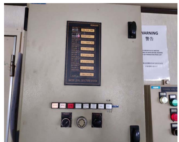
Water ingress alarm failure
