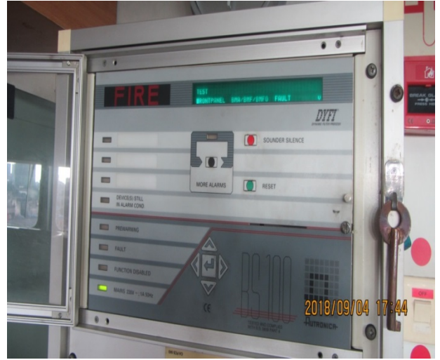
Fire detection and alarm system failure
