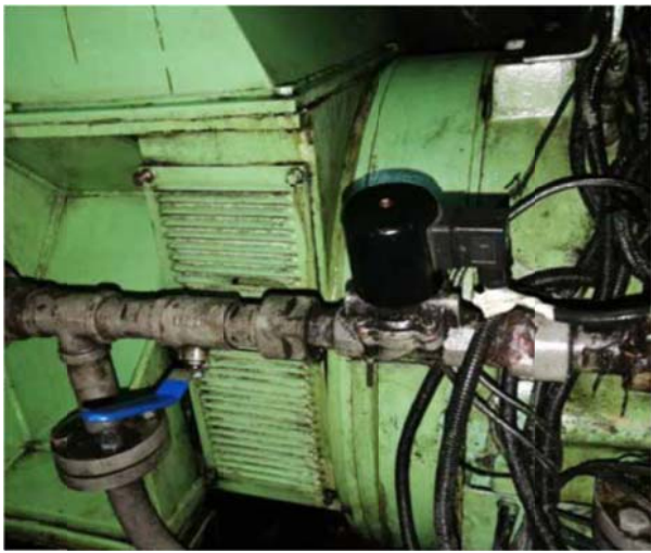
Starting air control valve of aux. engine failure
