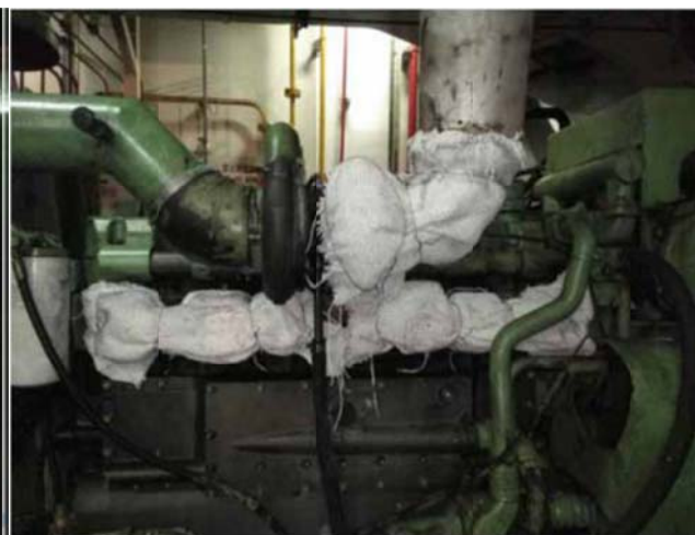
Exhaust pipe of Aux. engine leak
