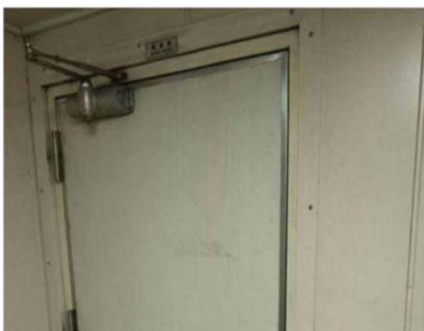
Self-closing fire door failure
