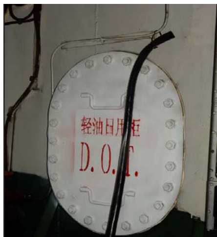
Oil leakage from the man hole cover of oil tan
