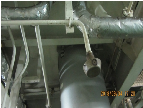
Local water mist fire fighting system failure
