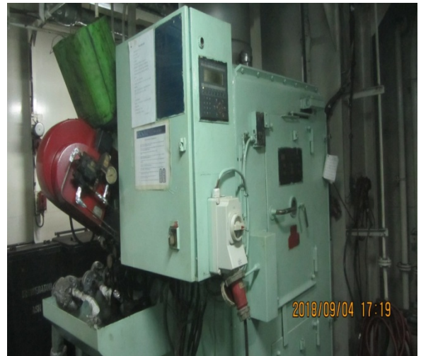
Incinerator igniting failure
