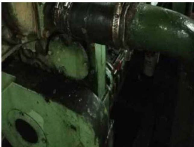
Sea water pipe of Aux. engine leak
