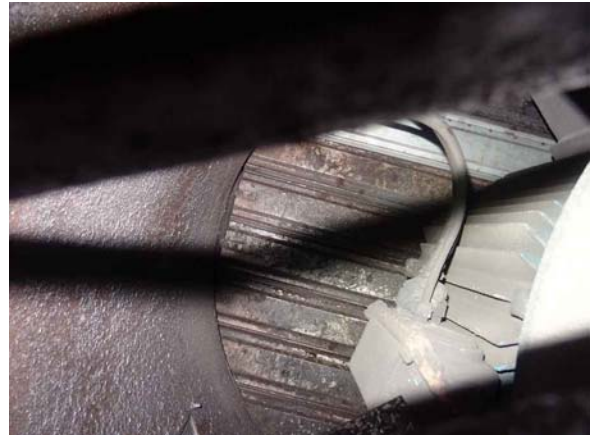
Fire damper of E/R ventilator damaged
