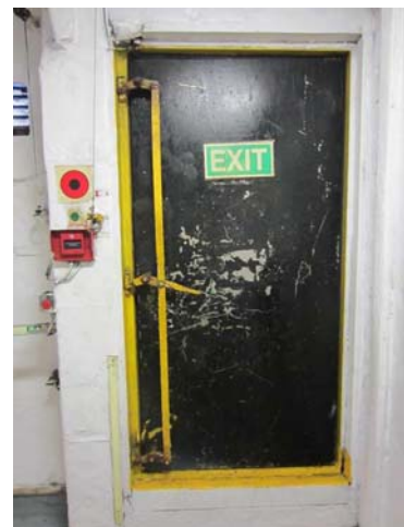
Weather-tight door on deck could not be closed.
