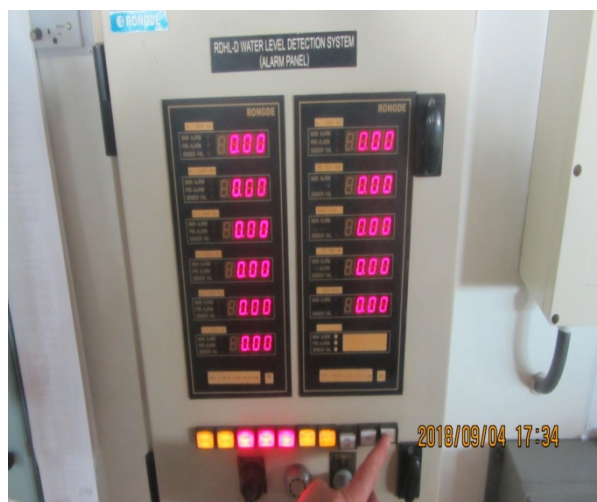
Water ingress alarm malfunction
