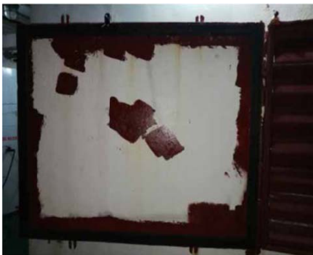
Cover of ventilator corroded
