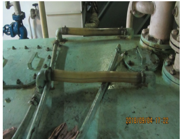
Re-flow pipe of STP was covered by paint
