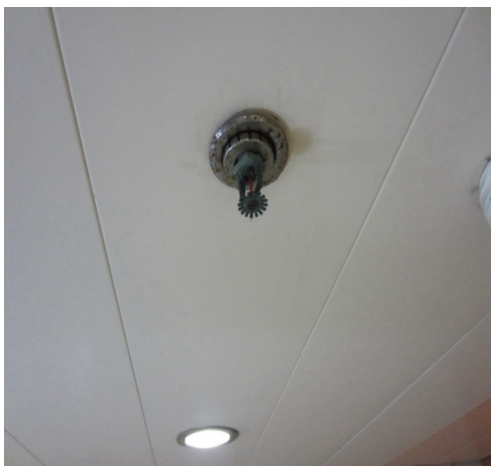
Water spray nozzle damaged.
