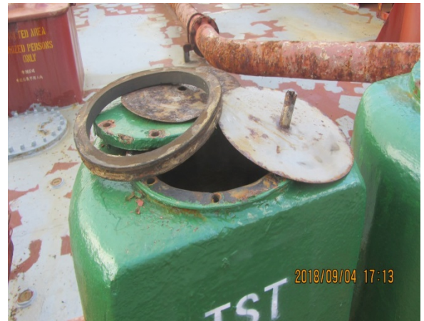
Air pipe head damaged
