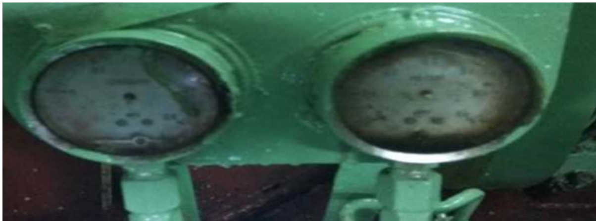
Sludge pump both pressure gauges are defective
