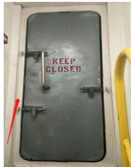
E.R. door not meet relevant reuirements.
