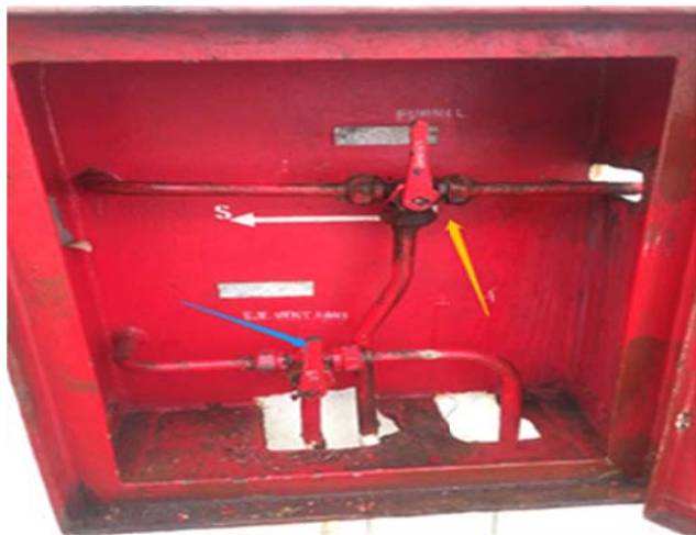
Funnel remote control pipe leakage
