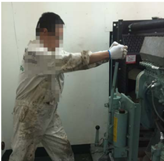
Emergency generator can not started by accumulator
