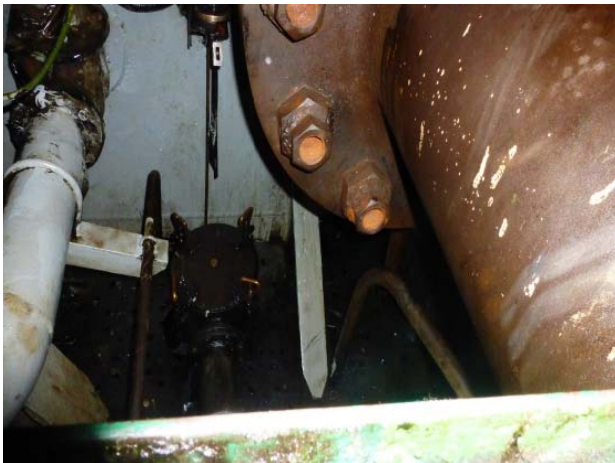
Main engine bottom oily seriously
