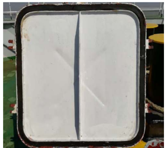
Hatch cover not watertight
