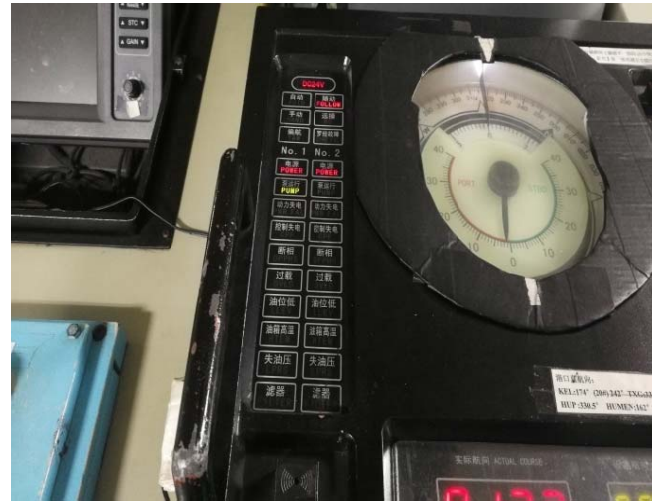
Steering gear alarm in wheel house without voice
