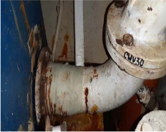
M/E Sea Water Cooling pipe Leaking
