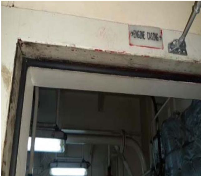
Seal of E.R. fire door damaged
