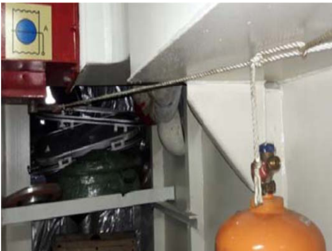
Fire damper at AC room obstructed by rope
