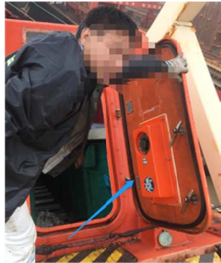
Rubber seals of of life boat door cracked
