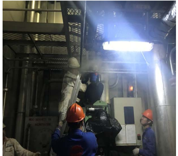
Local water mist system failure
