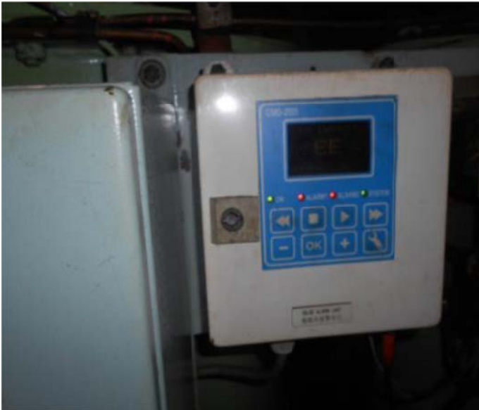
Oily water separator defective
