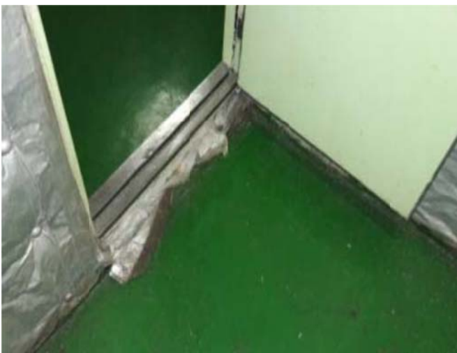
CO2 room entrance insulation broken
