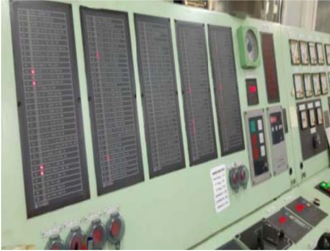
M.E. LO Low Pressure Defective
