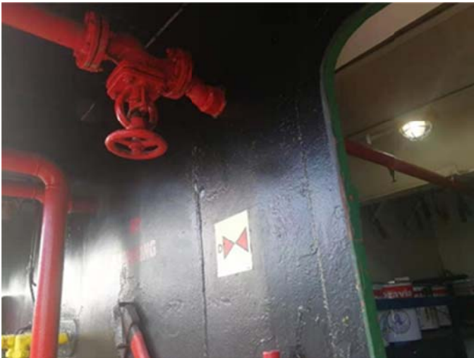
Paint store fire fighting system not properly marked
