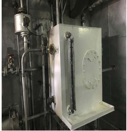
Steering gear oil tank low level
