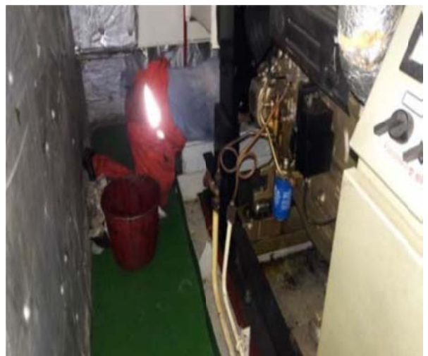
Emergency Generator oil leaking
