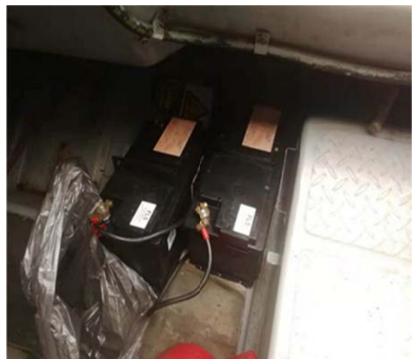
Lifeboat batteries out of order
