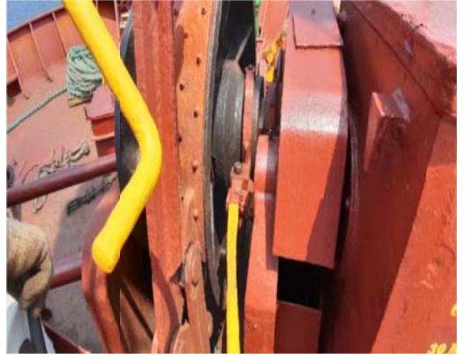
Safety pin of mooring winch unsecure
