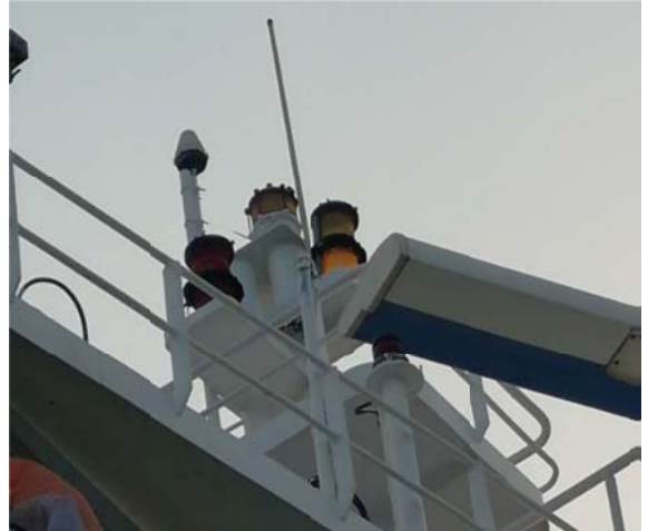
Navigation lights inoperative
