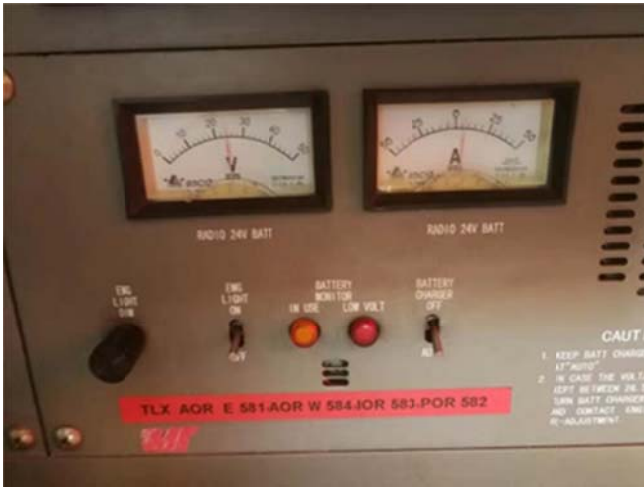
GMDSS reserve power indicator failure
