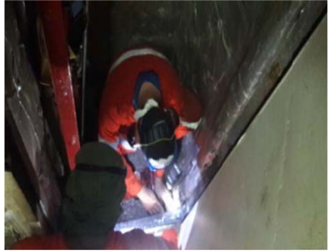
Escape trunk door corrosive, broken
