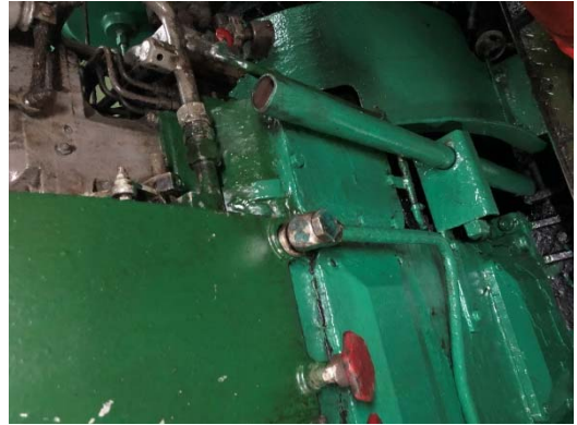
M.E. fuel oil leakage
