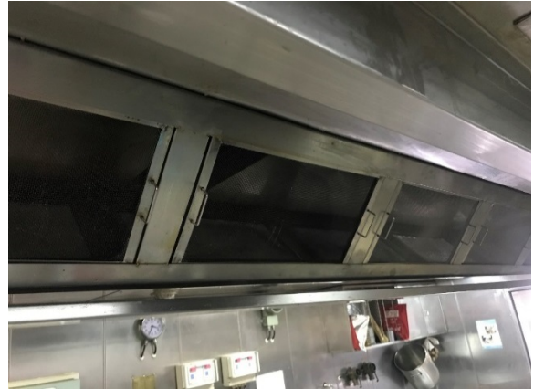
Galley exhaust ventilator filters dirty
