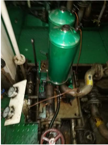
Auxiliary Engines oily
