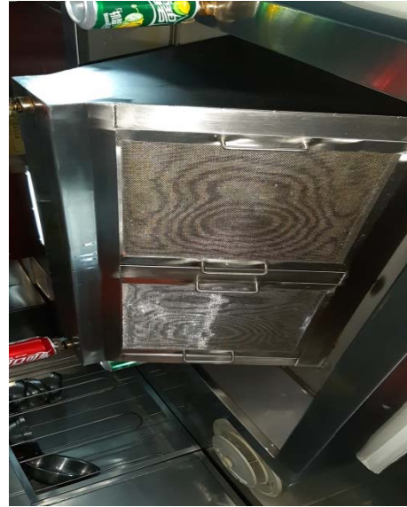
Air vent for galley room oily
