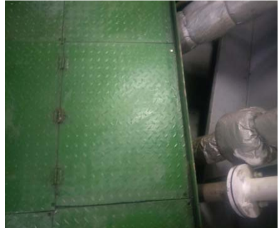
Some ER flooring plates not secured (rectified)
