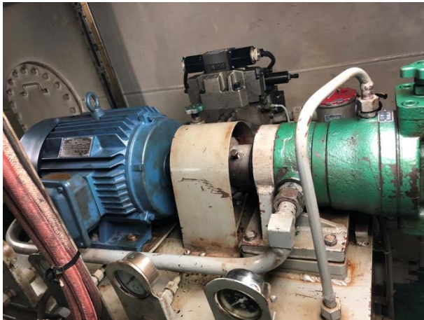
Pump shaft not protected by cover.
