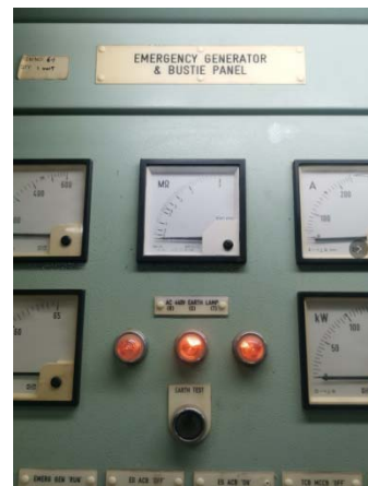
Emergency switch board low insulation
