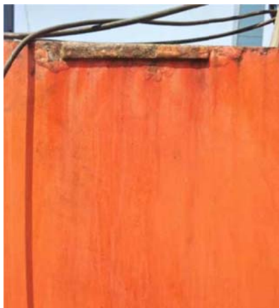
Deck line unclear painted
