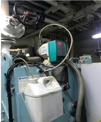
Disinfectant pump for sewage treatment plant inoperative
