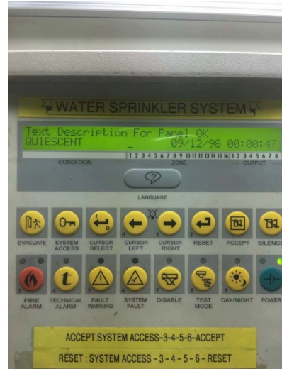
Water sprinkler system not working
