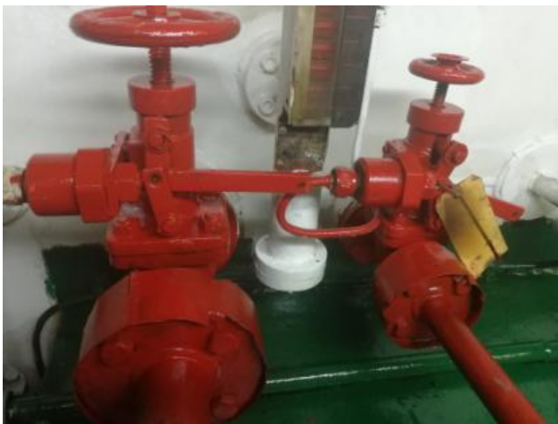
Quick closing valves leaking (rectified)
