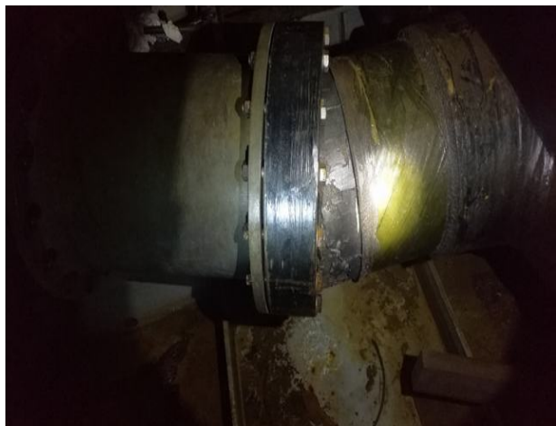
Water leakage of ballast pipe of pipe tunnel
