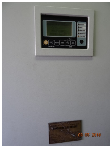
VDR damaged (already repaired)
