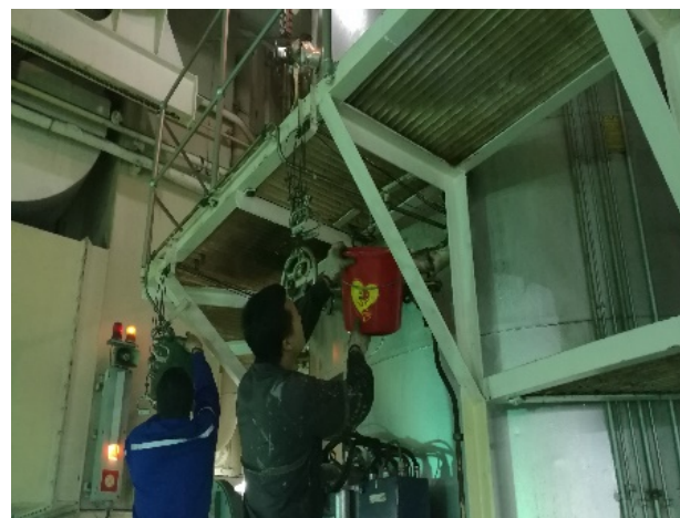
E.R. local water mist system failed
