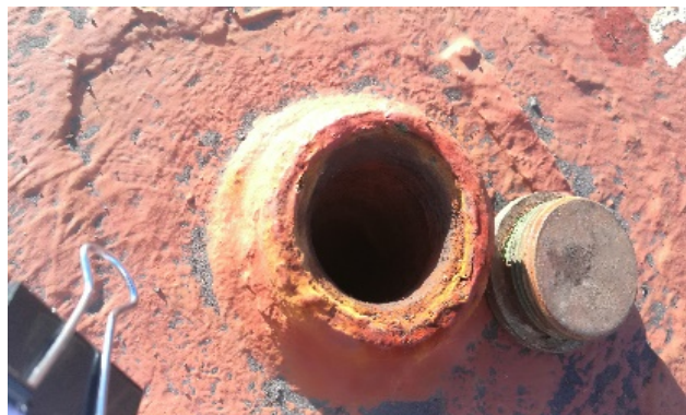
The cap for sounding pipe cannot be closed
