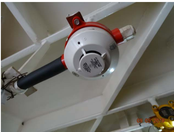
Fire detector in paint room damaged (already replaced)
