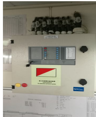
Fire detecting system in cargo hold failed
