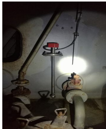
Water ingress alarm failed
