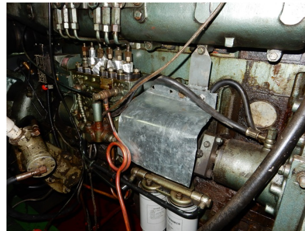
Protection cover of generator shaft lost (temporarily installed)
