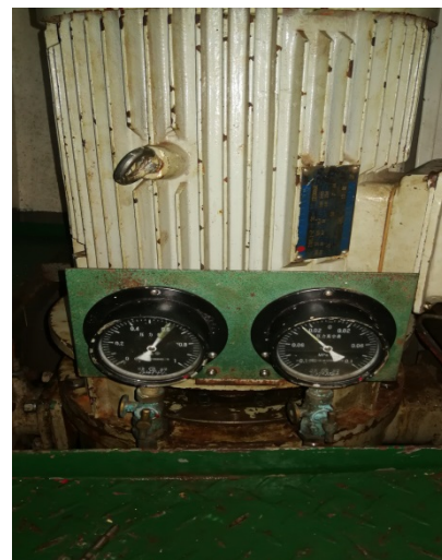
Test after restoration of emergency fire pump
