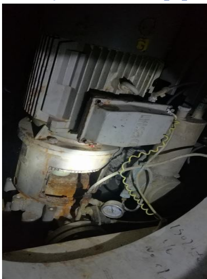
Emergency fire pump did not work
