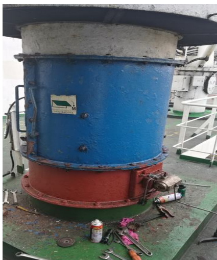
Damper of ventilator of engine room cannot be closed
