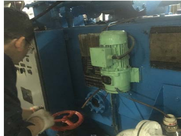
Chemicals supply pump of sewage water treatment plant failed
