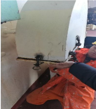
Gooseneck ventilator cannot be closed
