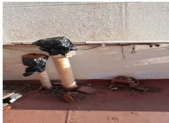
Poor condition of air pipe head
