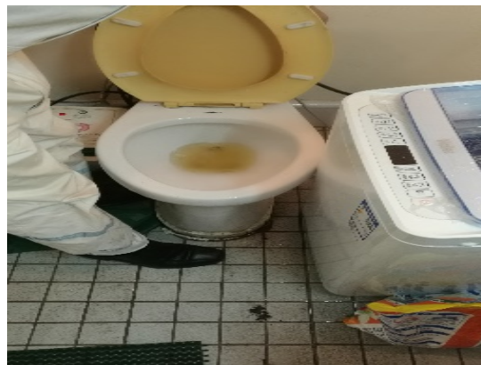
Untidy restroom, invalid flushing system
