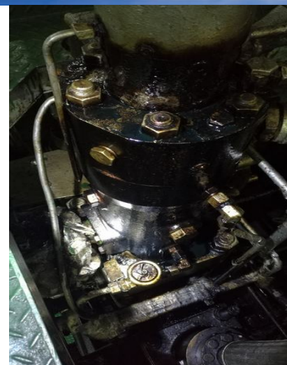
Oil leakage of high pressure oil pump
