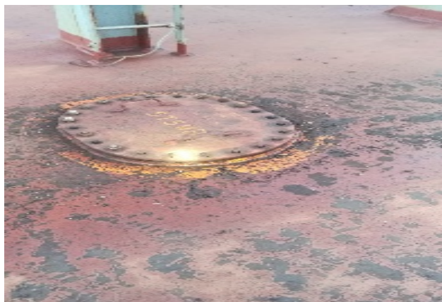
Invalid water tightness of manhole cover of ballast tank
