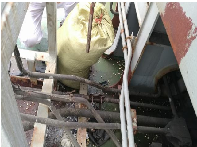
Leakage of hydraulic oil pipe on deck
