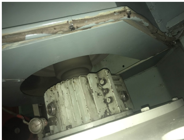
Cleaned bottom of auxiliary engine
