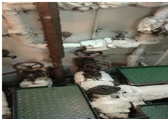
Low pressure of controlled air, and the quick closing valve cannot be closed
