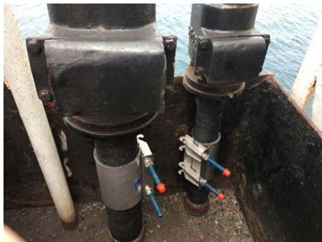
Corroded and holed air pipes
