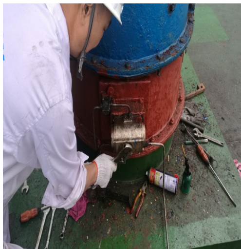
Fire damper on E.R. ventilator seized.
