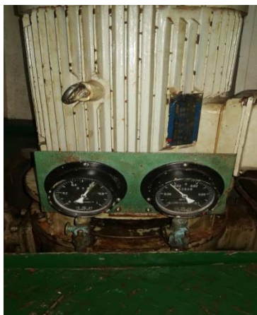
Emergency fire pump damaged
