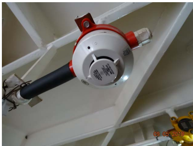
Fire detector in paint store damaged.
