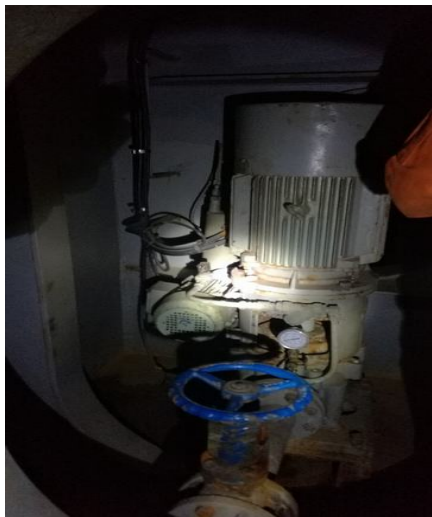
Emergency fire pump damaged.
