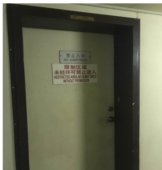
Self-closing fire door failure (rectified)
