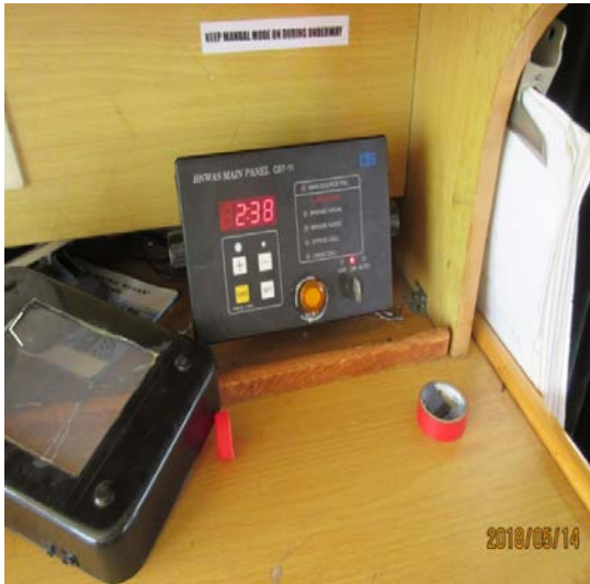
Crew members are unfamiliar with BNWAS operation.
