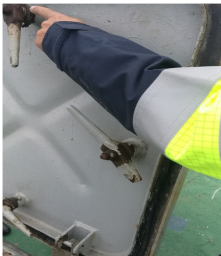
Small hatch cover for cargo hold could not be closed tightly
