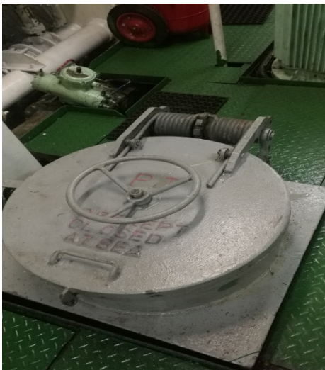
Pipe tunnel cover could not be open (water ingress)
