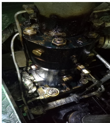
Oil leakage found from high pressure pumps.
