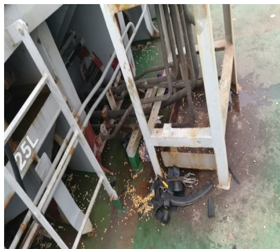
Oil leakage found from hydraulic oil pipe on deck
