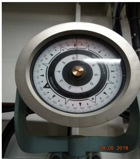
Gyro repeater in steer gear room failure.
