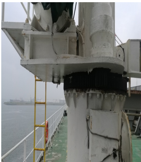
Limit switch on oil pipe crane missing
