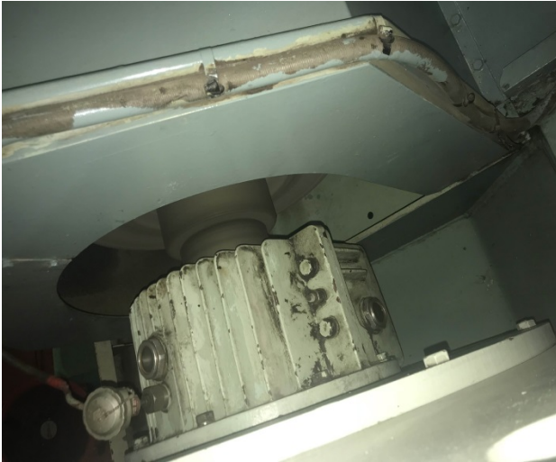
Aux. engine bottom oily (rectified)
