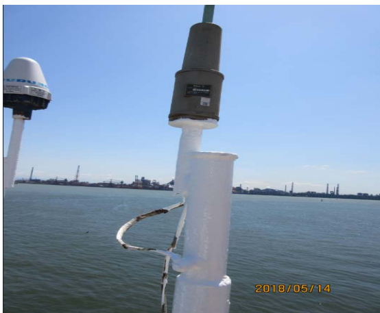
Antenna support post corroded
