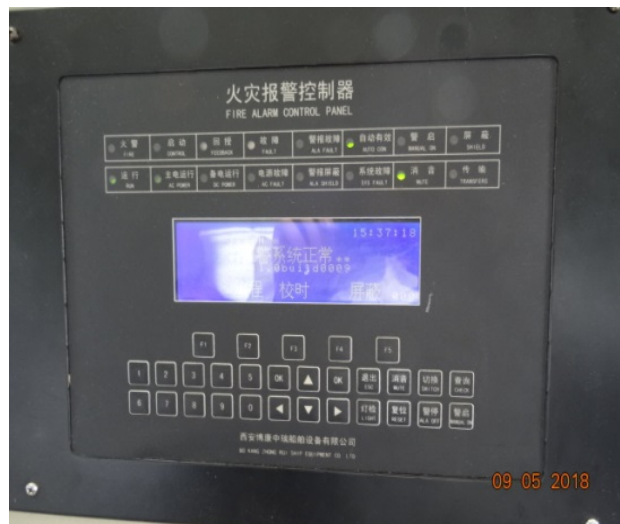
Fire detection alarm system damaged (rectified)
