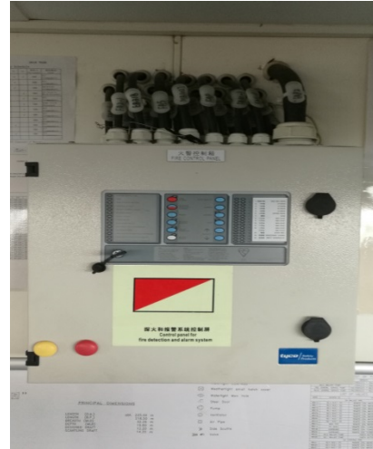
Cargo holds fire detecting system failure.
