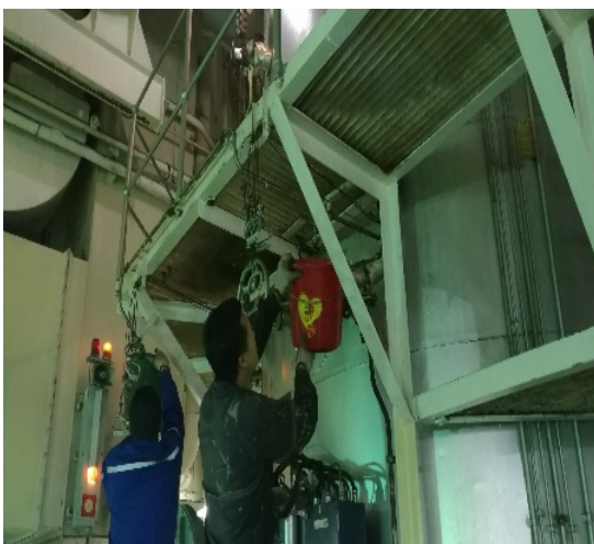
Local water mist system in Engine Room not working.
