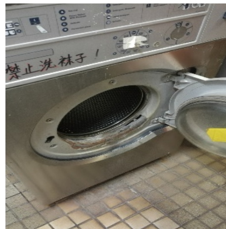
Washing machines (clothes) not operational or disconnected.
