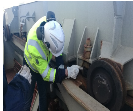
Automatic-cleats and Locking Bolts for hatch covers not fully functional due to seized / corroded.
