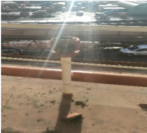
Air pipe head, poor condition
