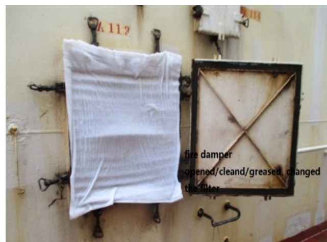
The hatch cover is seriously corroded and cannot be closed.
