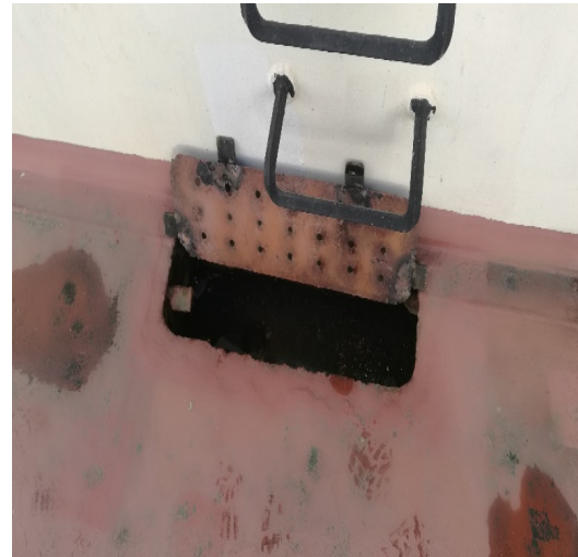
Supporters / stiffeners of deck plating missing
