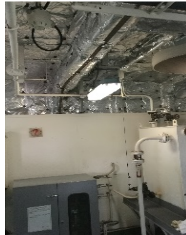
A large number of lighting lamp damage (has been repaired)
