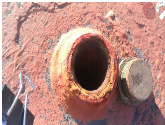
Several closing devices/plugs on main deck are not able to be closed.
