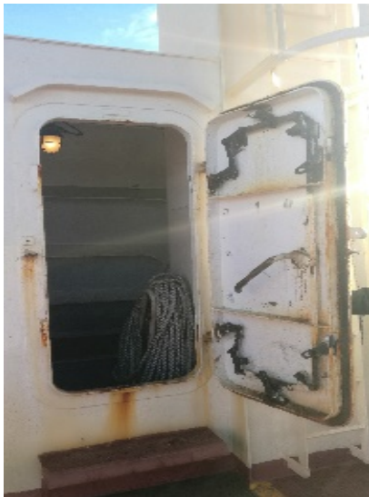
Watertight door forecastle is not able to be properly closed.
