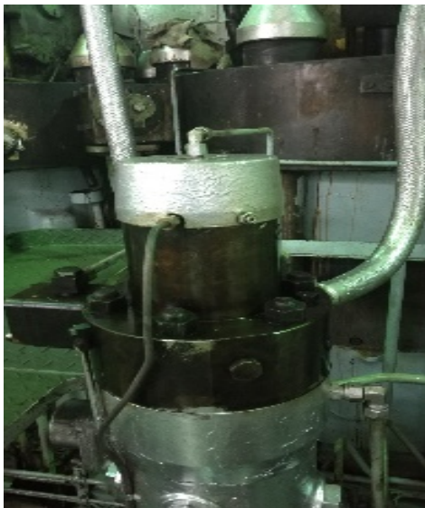
Main Engine high pressure fuel pump is leak large amount of fuel oil.
