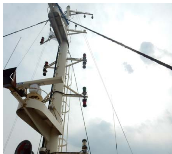
Radar mast support wire loose.
