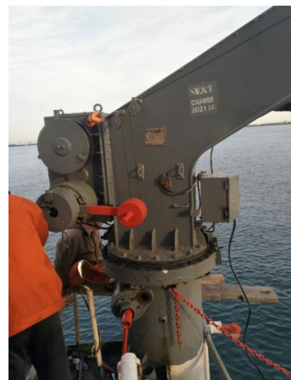
Rescue boat release device does not function properly.
