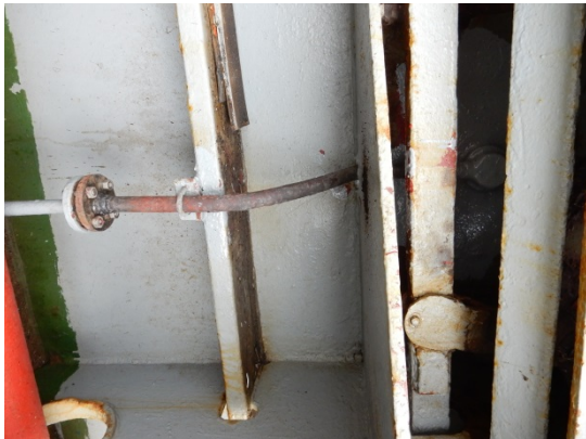
Pipe for fixed CO2 system on No.2 cargo hold holed.
