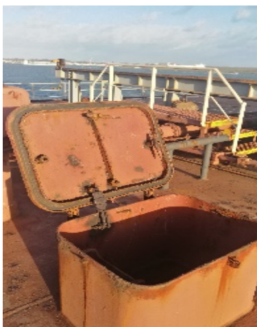
Small hatch cover plate of cargo manhole cannot be closed effectively.
