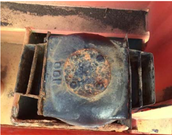
Vent aire pipes are corroded and damaged.
