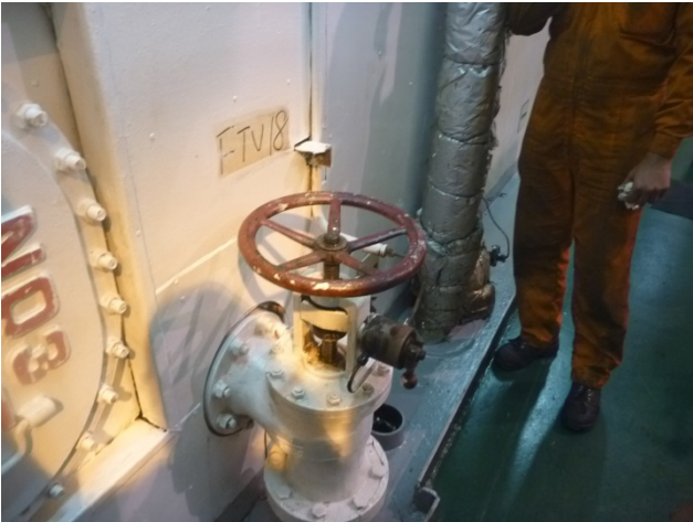
Quick closing valve of MGO cabin was blocked with a wood block (wood has been removed).
