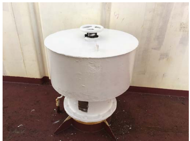
Ventilator can't be closed tightly.
