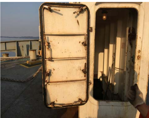
Weather tight door can't be closed tightly.
