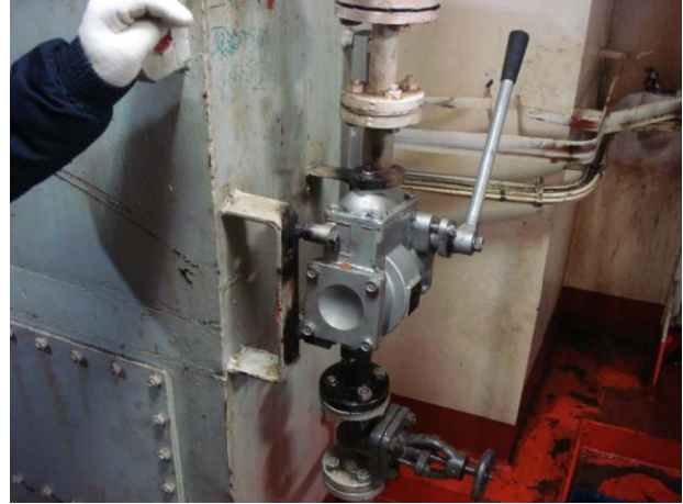
Hand pump leaks oil.
