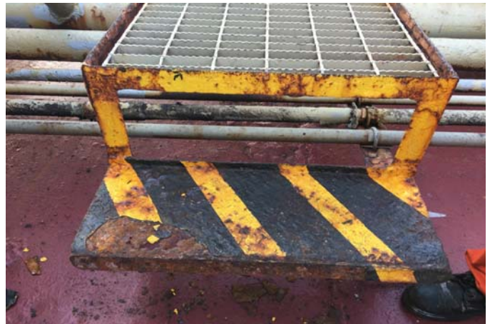
Footboard between cargo holds are rusted through.
