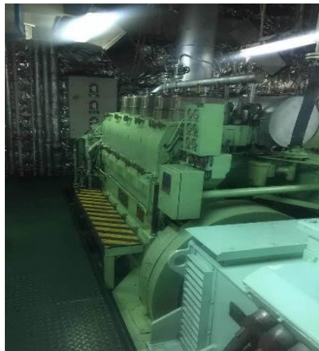
D.G High pressure pipe not covered
