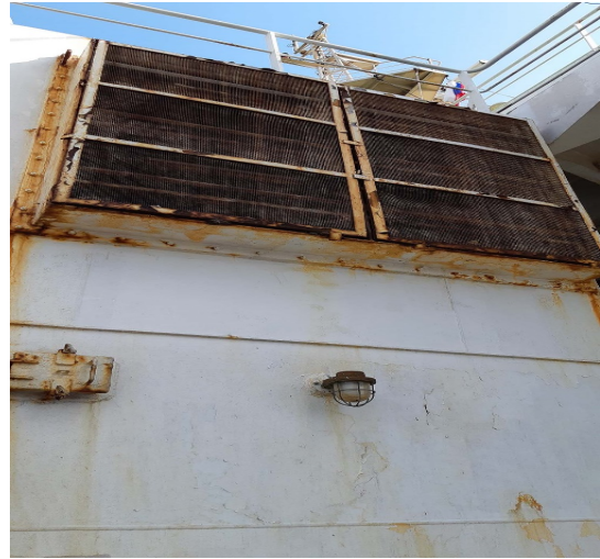
Engine room ventilation fire dampers corroded, damaged
