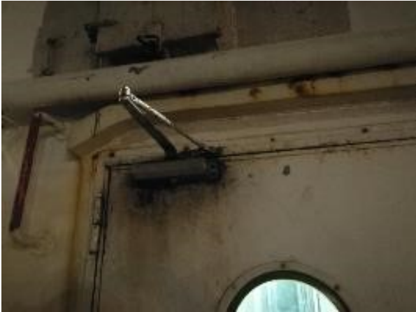
Fire door self-closing device damaged(rectified)
