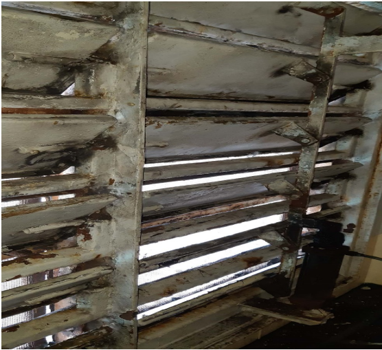
Engine room ventilation fire dampers corroded, damaged
