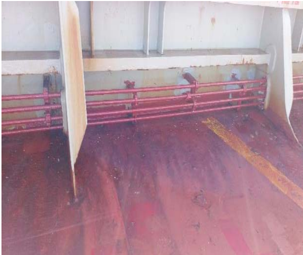
C.H. covers hydraulic piping badly corroded, clamps and brackets missing
