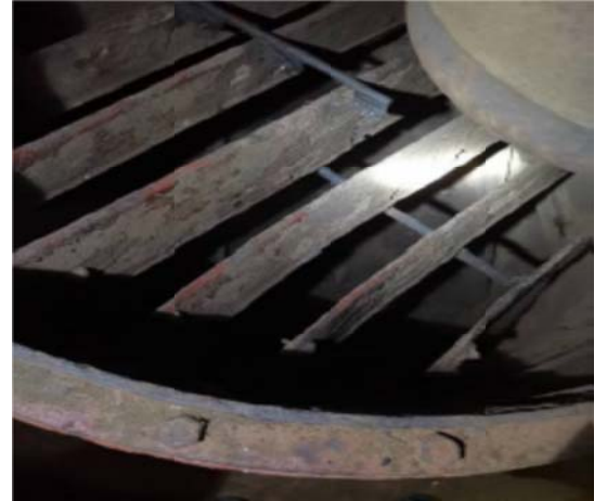
Engine room ventilation fire dampers defective.
