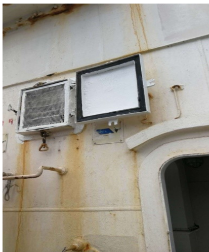
Ventilation cover of battery room corroded
