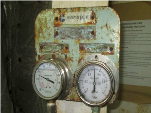
Water pressure of emergency fire pump not enough
