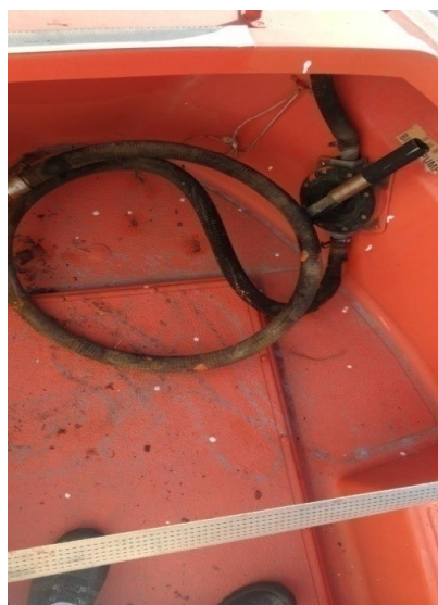
Rescue boat: pump suction pipe not connected
