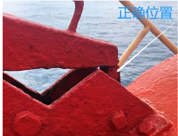
Free fall lifeboat release system defective (rectified)
