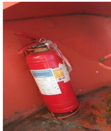
Rescue boat: fire ext. not fixed
