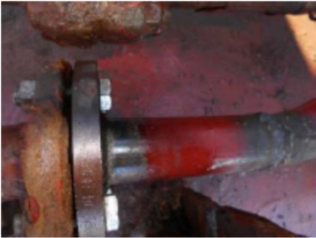
Winch hydraulic oil leaking
