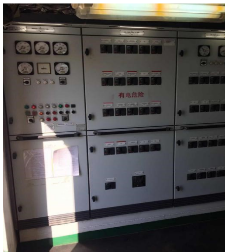
EM D.G unofficial cables connection (rectified)
