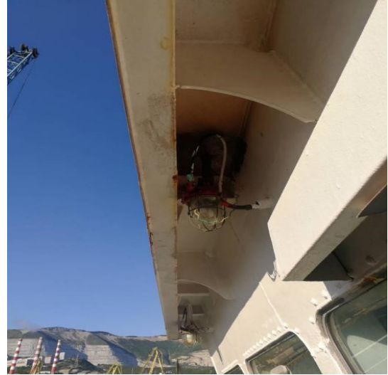
Emergency lighting fastening pipe corroded
