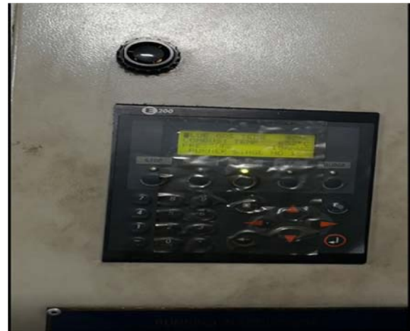
Incinerator defective( below 650°C starting over 5 minutes )
