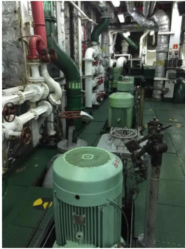
BW pump case leak
