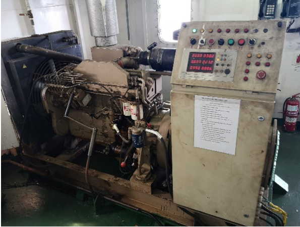
Auto start emergency generator has failed test.
