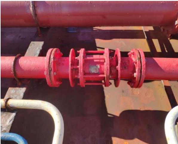
Leakage noted from expansion joints at fire main on deck
