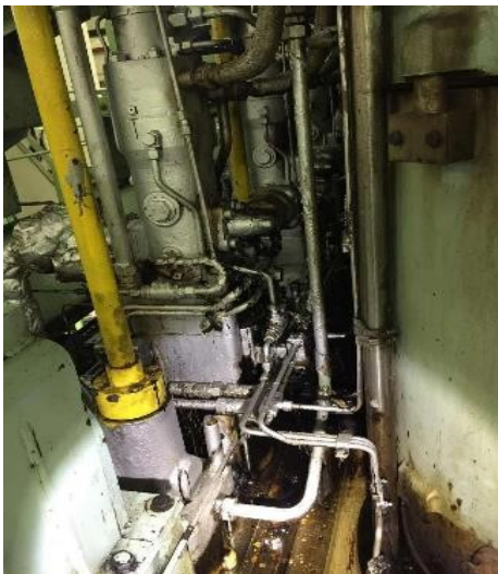
Fuel oil booster pump shaft seal leak
