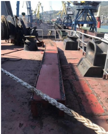
Stern mooring winches walkway (steel) corroded
