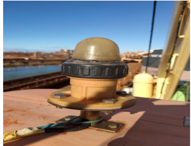
Rescue boat canopy light defective
