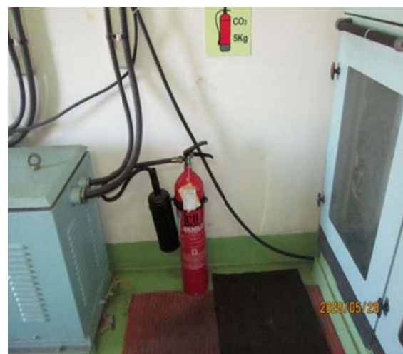
Portable fire extinguisher not near the entrance of E.G. room
