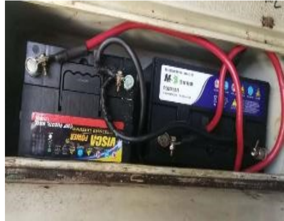
Life boat batteries no power (after renewal)
