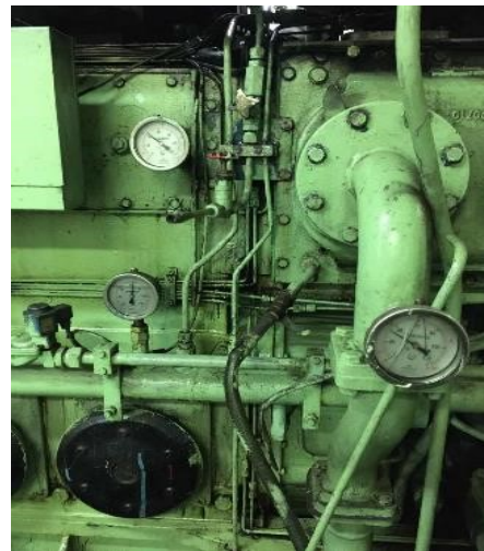
D.G heavy leak of oil
