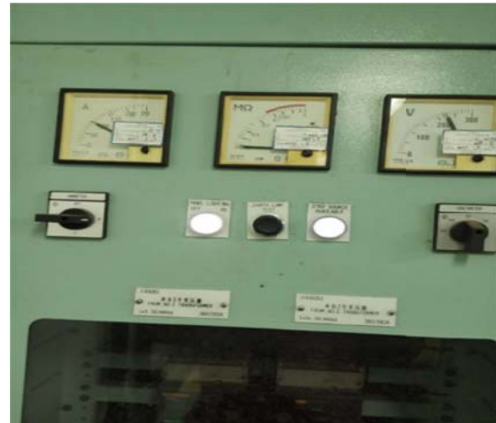
Emergency switch board 了ow insulation
