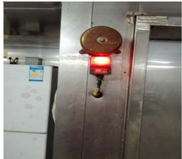
Cold rooms (Reefer chambers) locked in alarm not operational (rectified)
