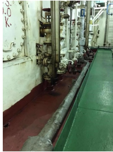
Oil tank in ER measuring glass leak
