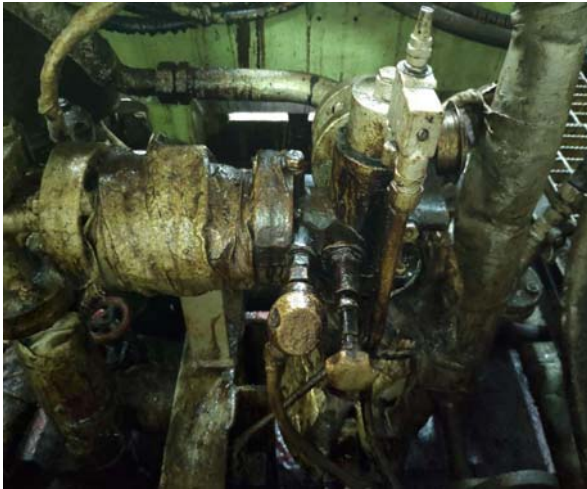
Several oil leakages and oily rags sighted in purifier room
