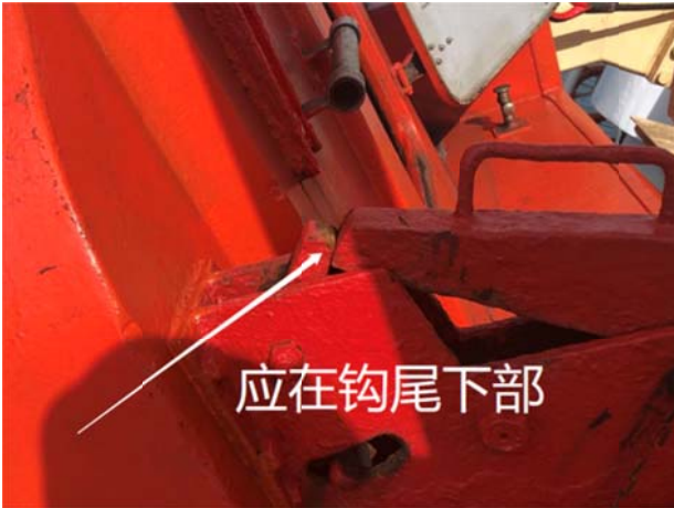
Free fall lifeboat release system defective.
