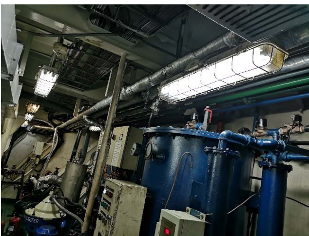
Lights of E.R. unlit(rectified)
