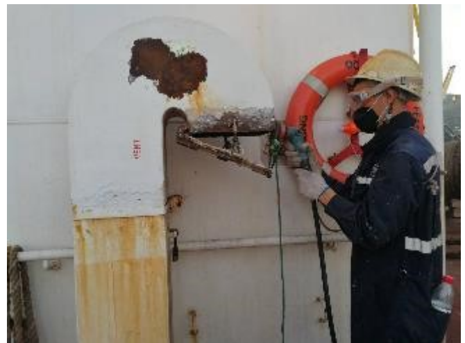
Ventilation cover corroded
