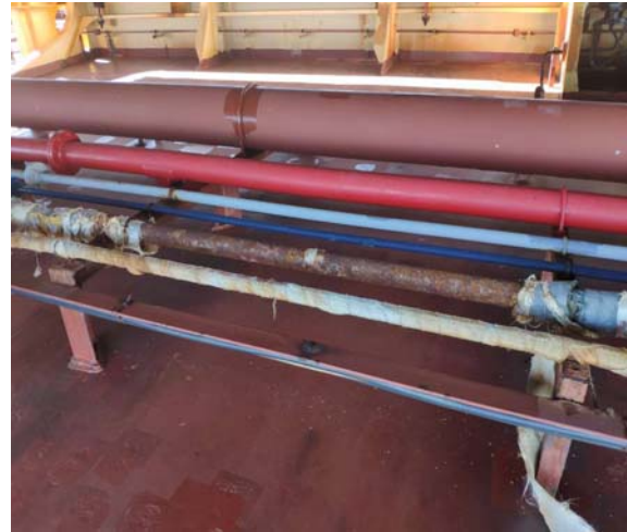
Insulation lagging missing at steam pipe on deck
