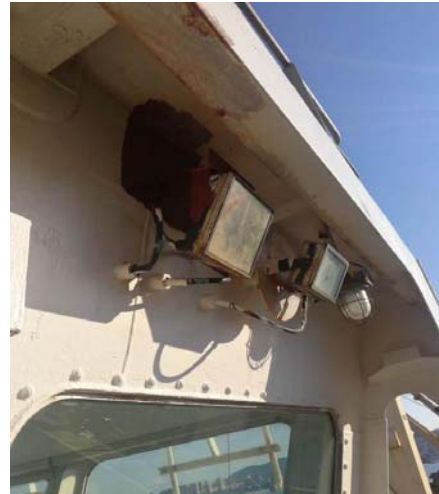
Revolution counter foundation heavy corroded
