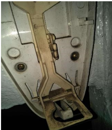
EPIRB bracket fixed not as required (one bolt)
