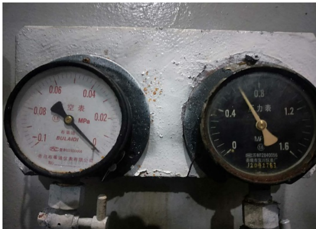
Emergency fire pump defective
