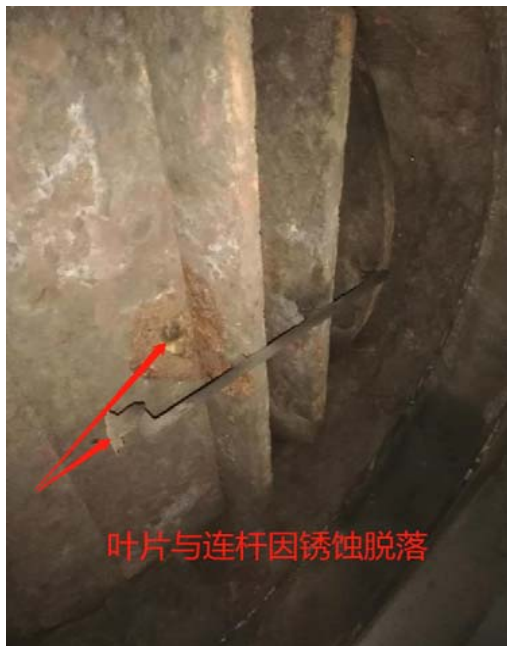
Connecting rod of fire dampers corroded and broken
