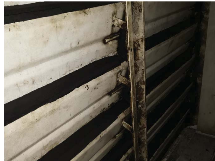
Air vent damper to E/R Port/ Stbd. not close properly
