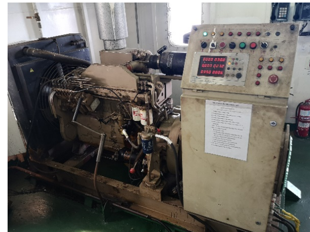
Auto start emergency generator had failed test
