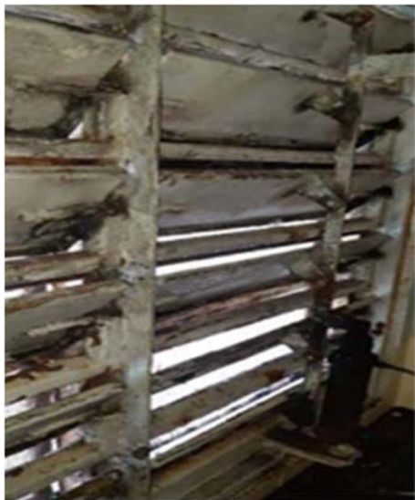
engine room grids corroded, damaged
