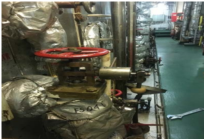
QUICK CLOSING V/V NOT ACTIVATED DURING TEST
