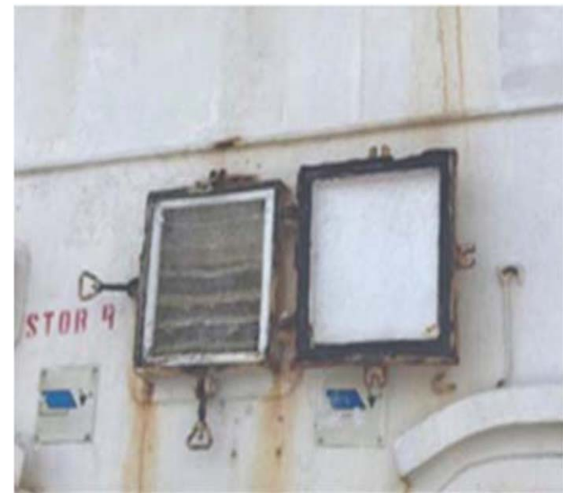
system of battery room ventilation cover corroded
