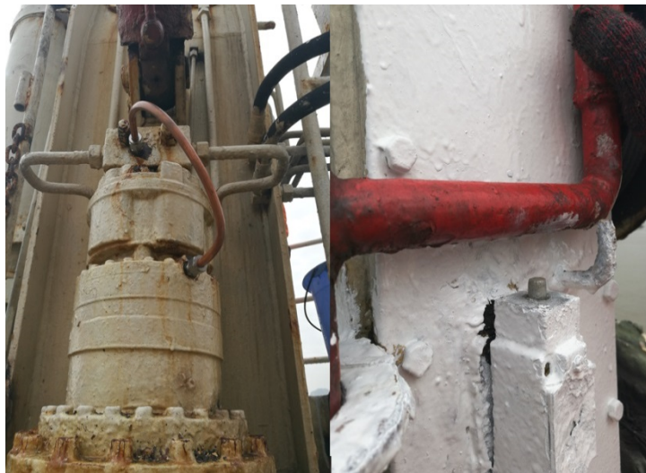
rescue boat davit hydraulic oil leakage ,limit switch malfunction
