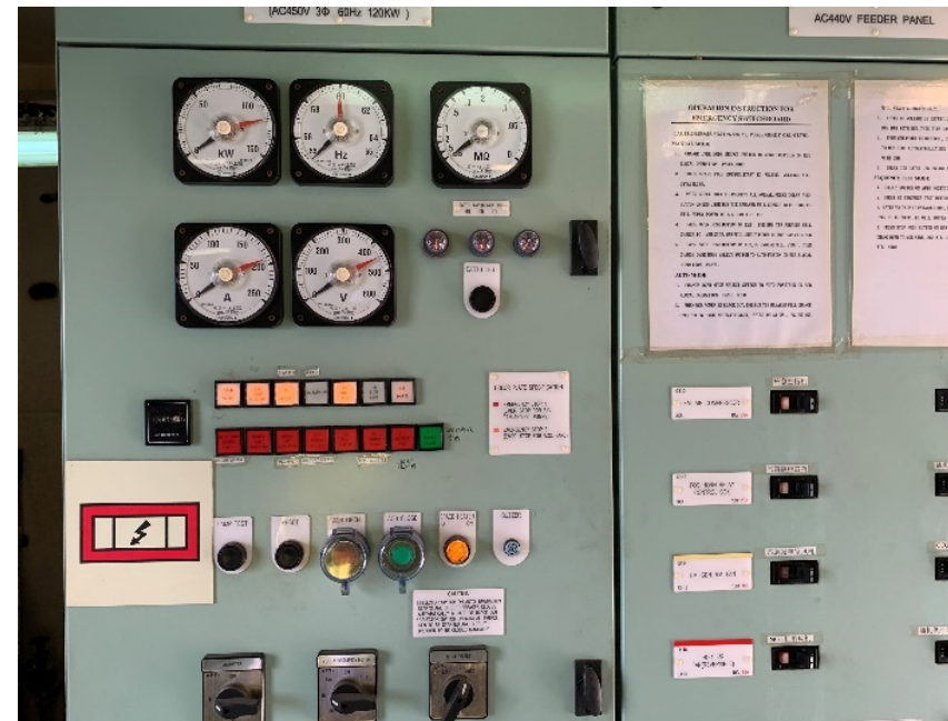
Emergency generator will not connect to emergency switchboard automatically
