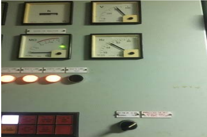
EMERGENCY GENERATOR--NOT STARTED DURING BLACK-OUT TEST
