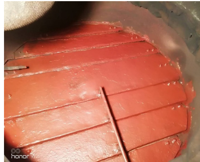
fire dampers deformed ( rectified)
