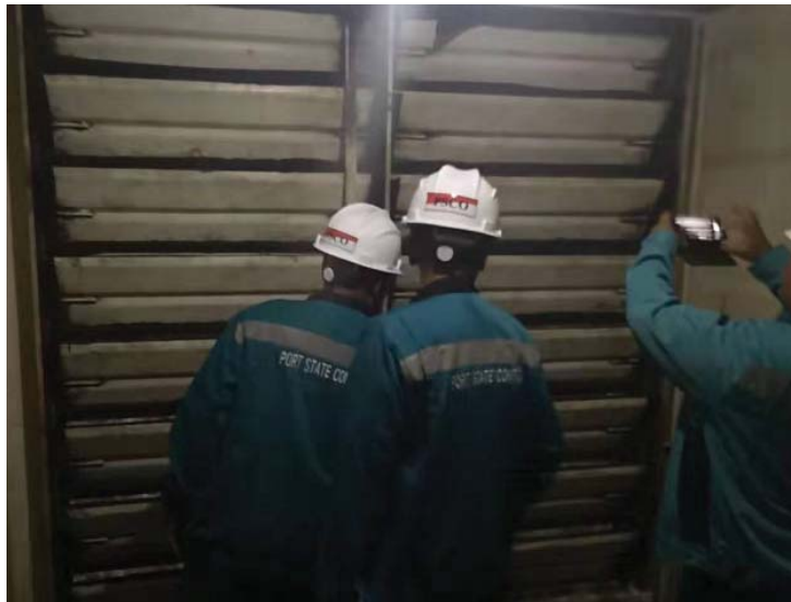
Fire funnel damper to E/R not close properly
