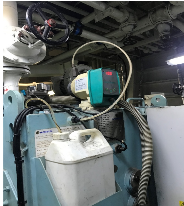
Disinfectant pump for sewage treatment plant inoperative
