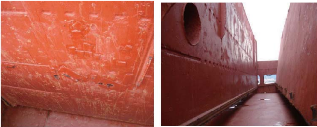
4-1 Holed hatch covers, attention to be paid to the lower part of the cover panels and the ventilators or cement holes in panel (if any)
