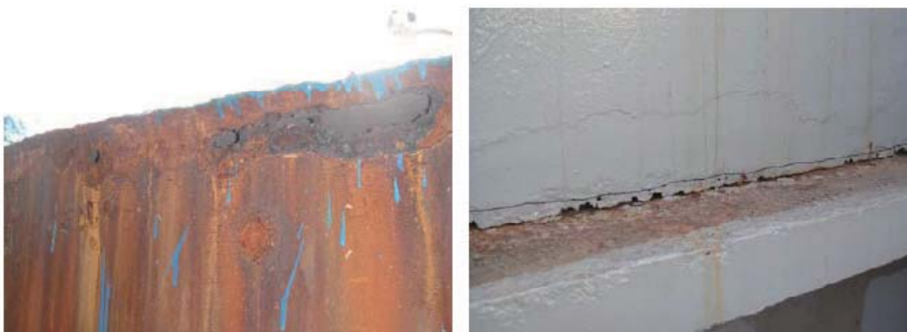
4-3 Seriously corroded skirt plate
