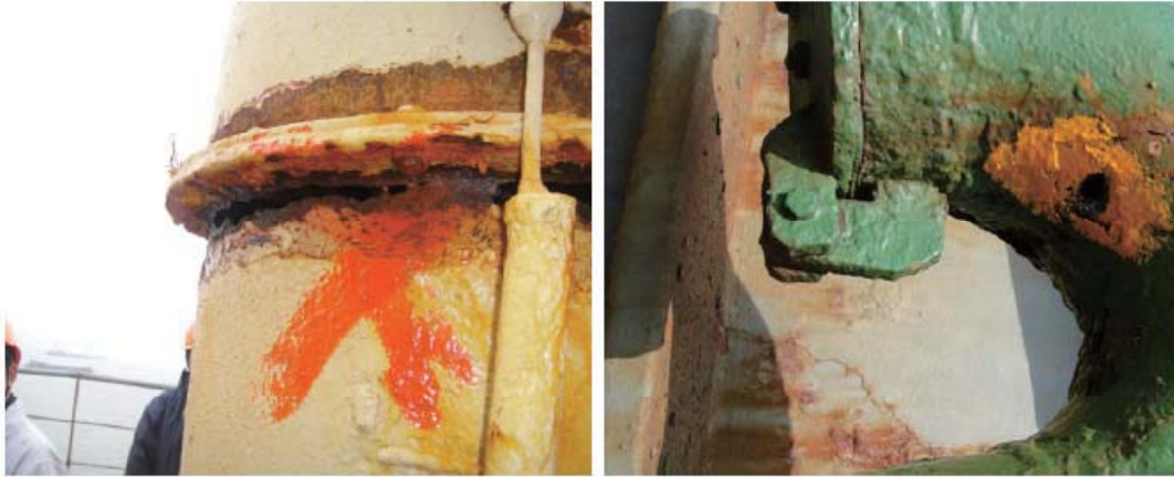
Figure 6 Holed ventilator and air pipe
