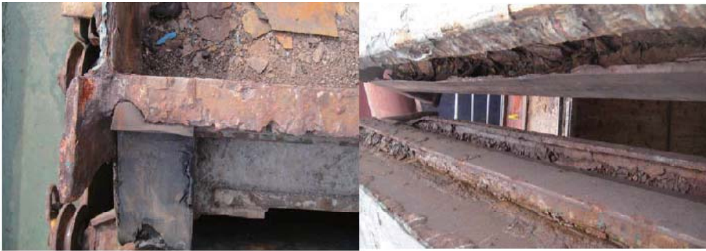
4-2 Seriously corroded rubber channel and draining channel
