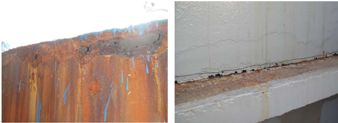
4-3 Seriously corroded skirt plate
