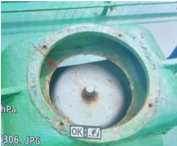
Top sealing ring missing
