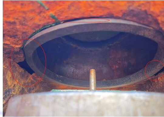
Corrosion and cracking of the top sealing ring groove
