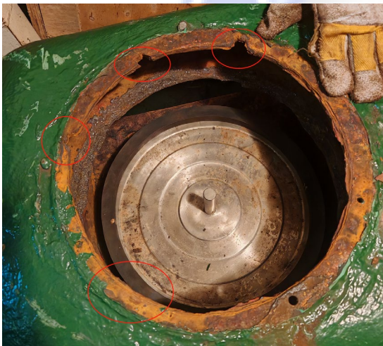
Cover plate bolt holes wasted due to corrosion
