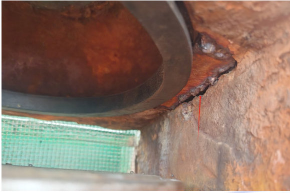
Cracking of the internal structure adjacent to the top sealing ring
