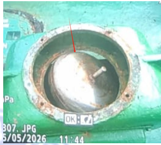
Missing sealing ring and detached float disc
