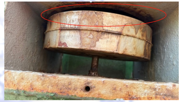
Float disc unable to achieve proper sealing
