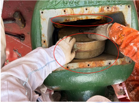
Sealing rubber ring missing, detached float disc
