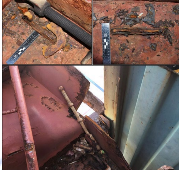
Figure 1: Thinned, heavily wasted and failed lashing eyes (top) and wasted and failed container support structure (bottom)
