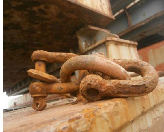
Serious Corrosion and Damage of Securing Parts and Components
