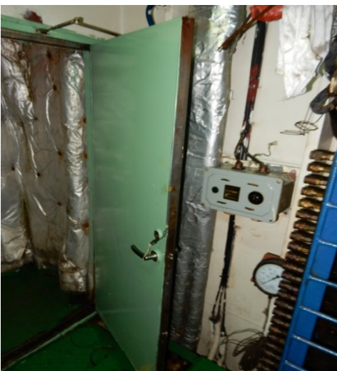
A60 Fire Door for Escape Tunnel Fastened by Ropes at Open Status
