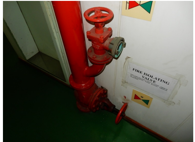
Crew Members Not Familiar with Position of Isolating Valve for Fire Main Pipe
