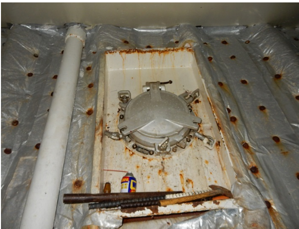
Failure to Close Storeroom Deadlight due to Rusting
