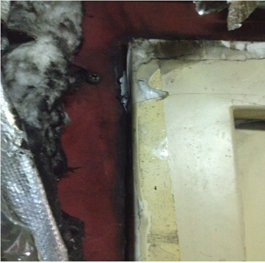
Light Coming from Gap between Fire Door Frame and Bulkhead (Riveted Door and Bulkhead)
