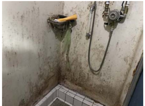
The bathroom of some crew rooms is of poor hygiene
