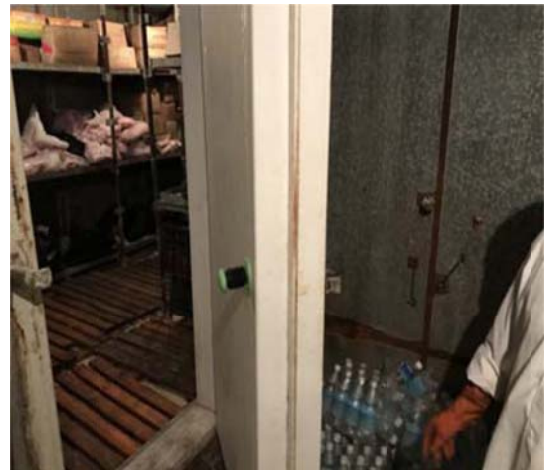
Failure occurs to the escape system inside the cold storage door (i.e. the opening device inside the cold storage door)
