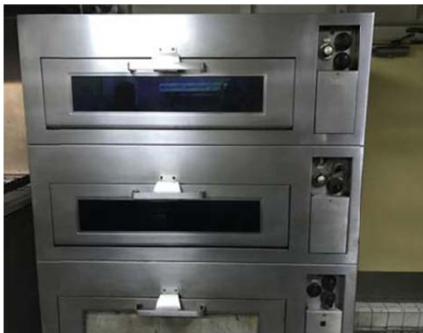
Failure occurs to the electric oven in kitchen
