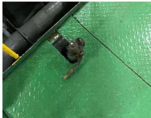
The self-closing device at the measuring hole of oil tank at the bottom of engine room is fixed in open position
