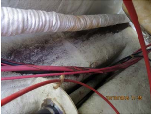
Hook release cable at the lower part of baseboard inside the lifeboat damaged.
