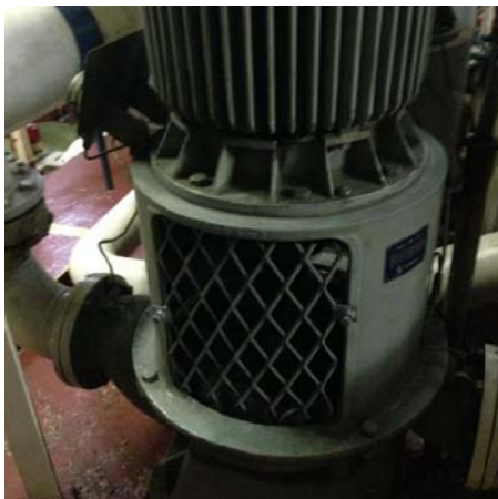
The low-temperature fresh water pump of the main engine has no safety protection (protecting net has been provided)
