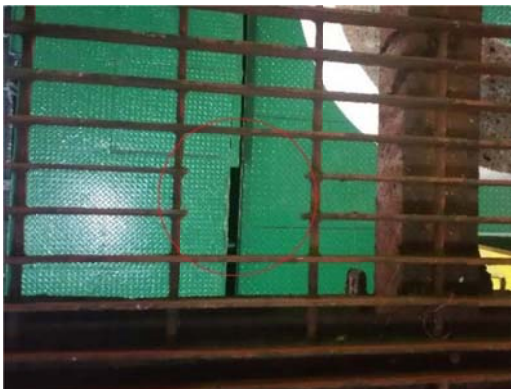
Two pieces of bars in the grille on the passage are missing
