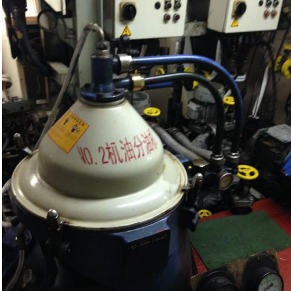
Serious oily under the oil separator
