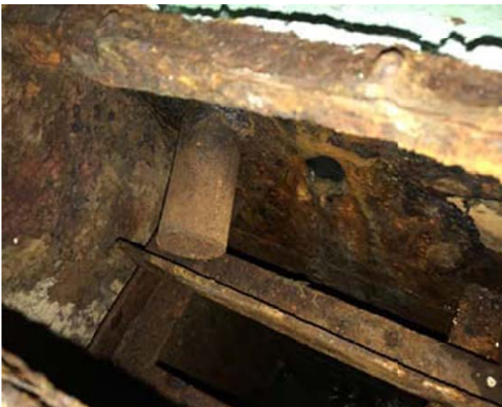
The wallboard in sewage treatment equipment is holed and serious corrosion.
