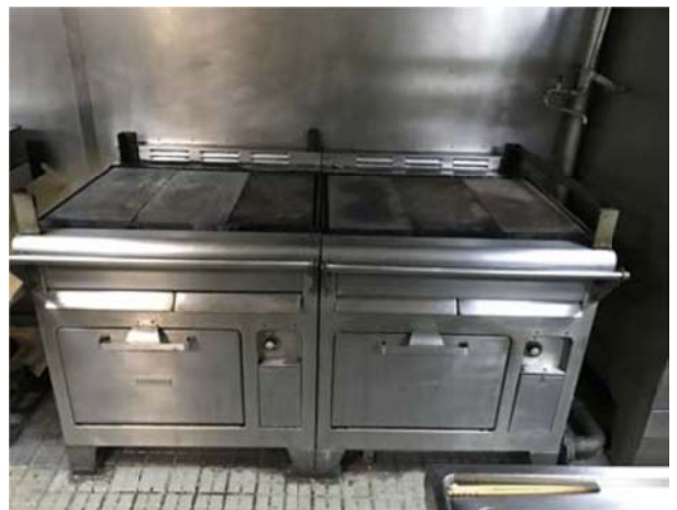
Failure occurs to the hot plate in kitchen
