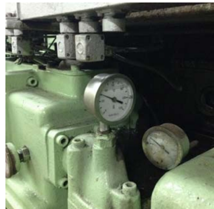
The generator instrument is damaged (already replaced)
