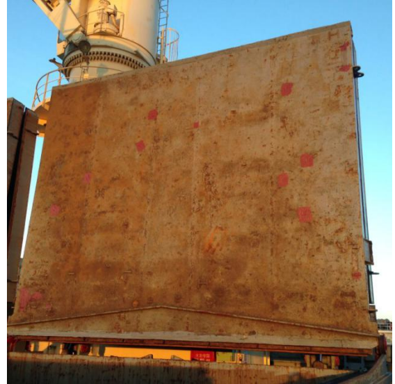
The hatch cover is seriously corroded
