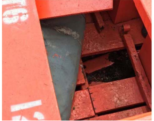
The pedal and plate inside the lifeboat get loose and rotten
