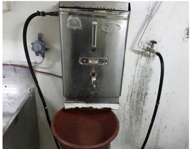
Failure occurs to the electric water heater in pantry
