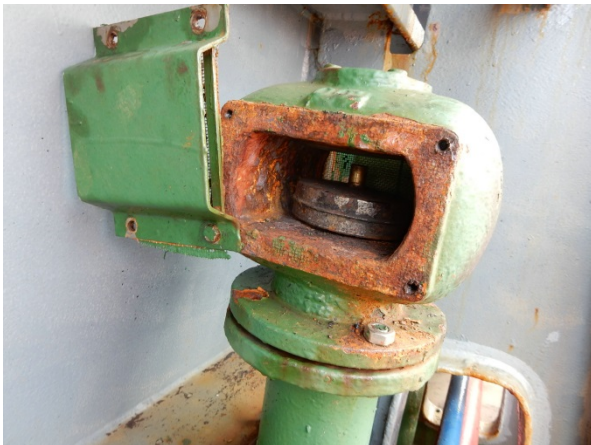
Float inside the air pipe head isn't active
