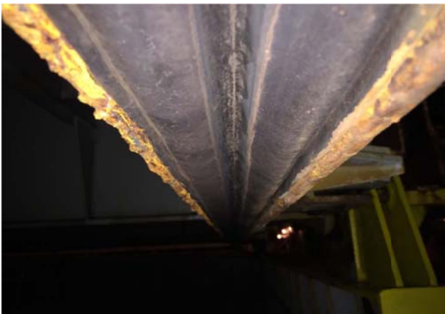
Sealing rubber strip of hatch cover is found with permanent
