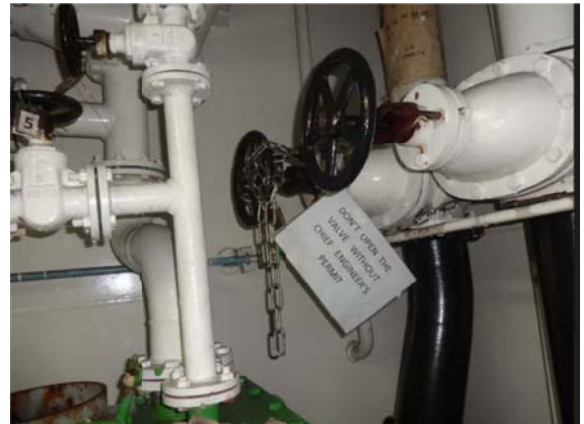
Sewage discharge valve is closed in the open position when the ship is within the port
