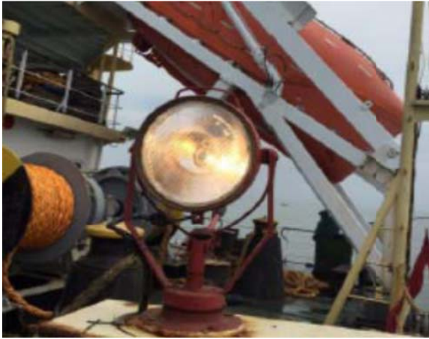
Emergency lighting does not work (repaired)
