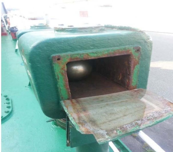
Air pipe heads malfunction
