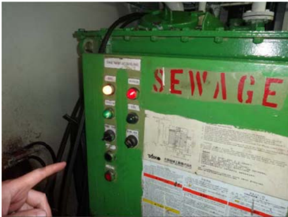
Sewage treatment unit hasn't been used for a long time
