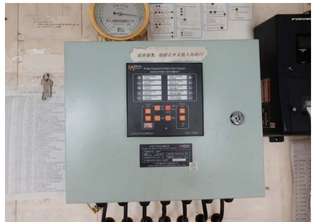
Crew members are not familiar with BNWAS operation
