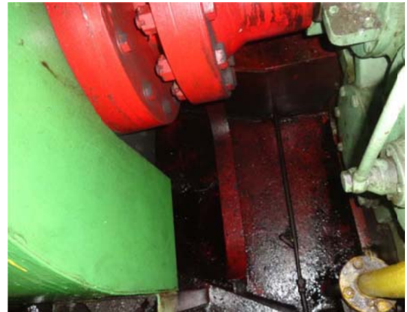
Heavy oil stains exist on the bilge
