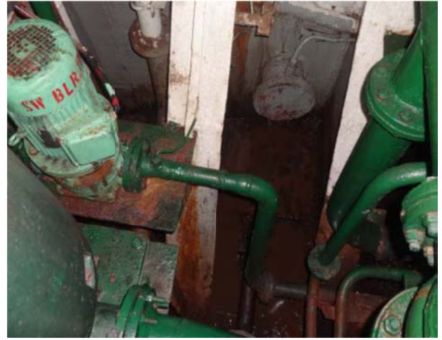
Water pump leaks
