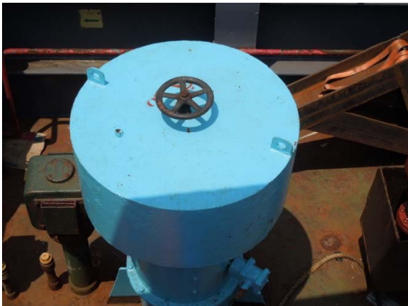
Ventilator cannot be closed
