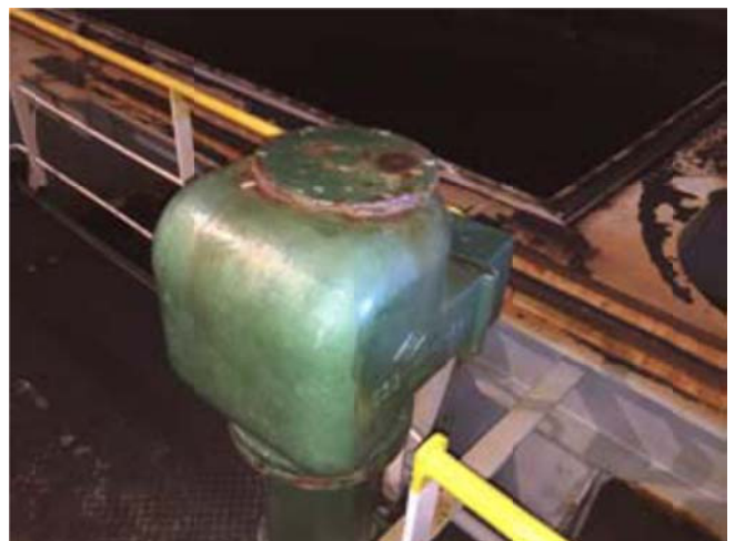
Cover on the top of air pipe head is corroded heavily
