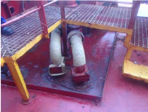
Oil from drip tray of mooring winches leaks through the oil drain plug
