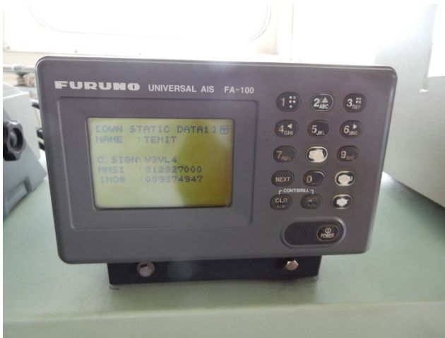
Crew members are not familiar with AIS operation
