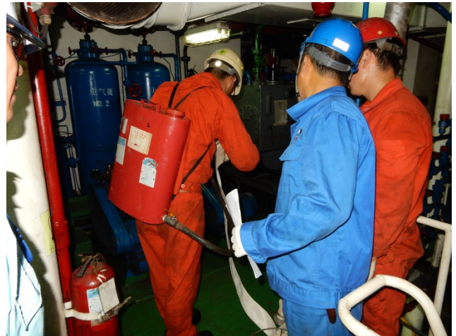
Crew members are not familiar with operation of foam extinguishing equipment
