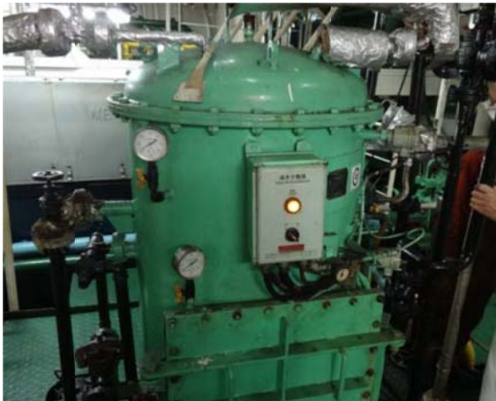
Oil-water separator of engine room hasn't been used for a long time
