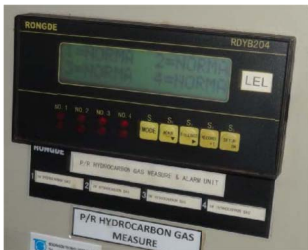
Pump gas detectors malfunction
