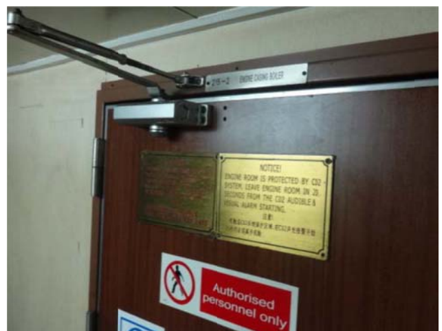
Fire-resisting door cannot be closed
