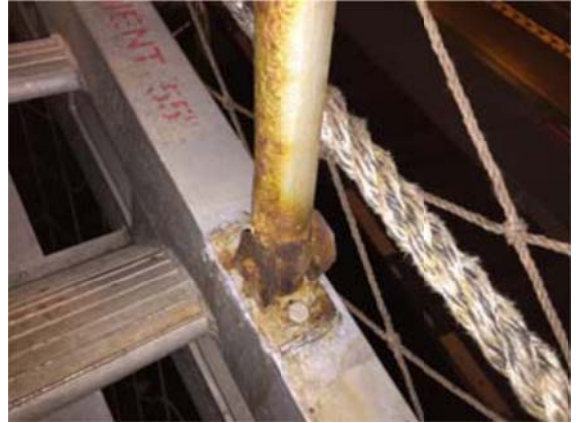
Corrosion exists at the column root of accommodation ladder
