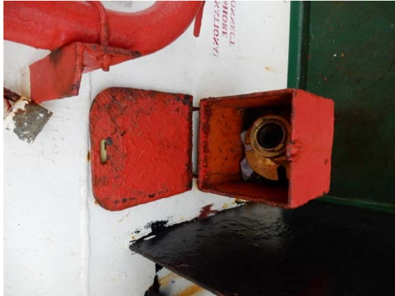
International shore connector for fire-fighting is not placed in the right position (rectified)
