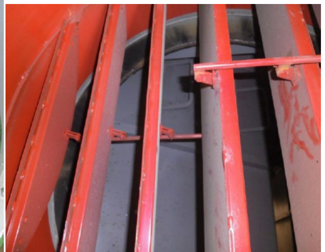
Figure 6: fire damper opened
