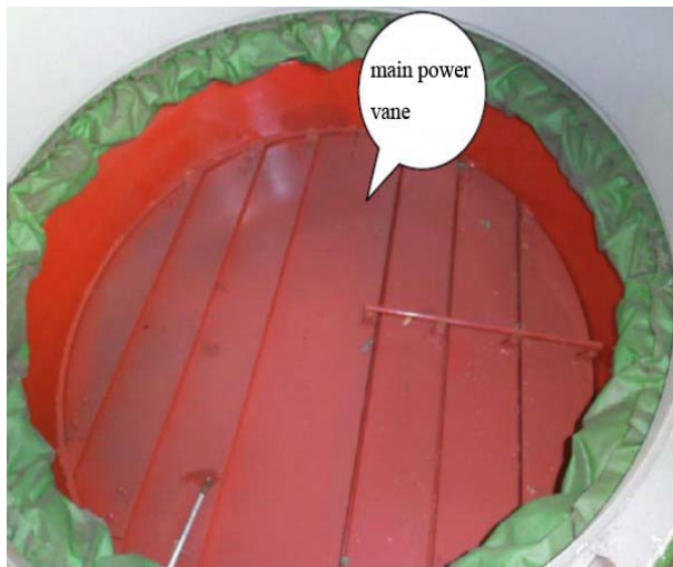
Figure 5: fire damper closed
