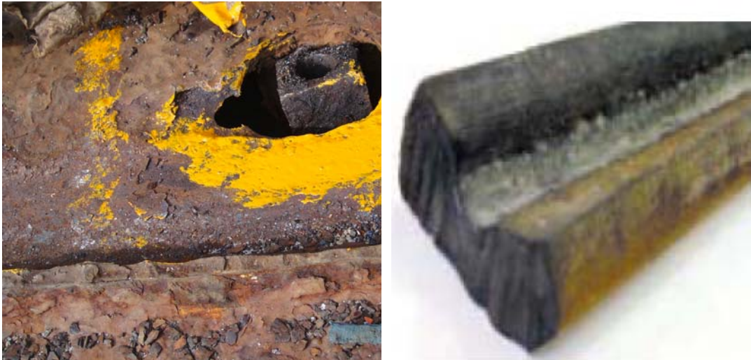
4-5 Holed face plate around cleat and over-compressed rubber
