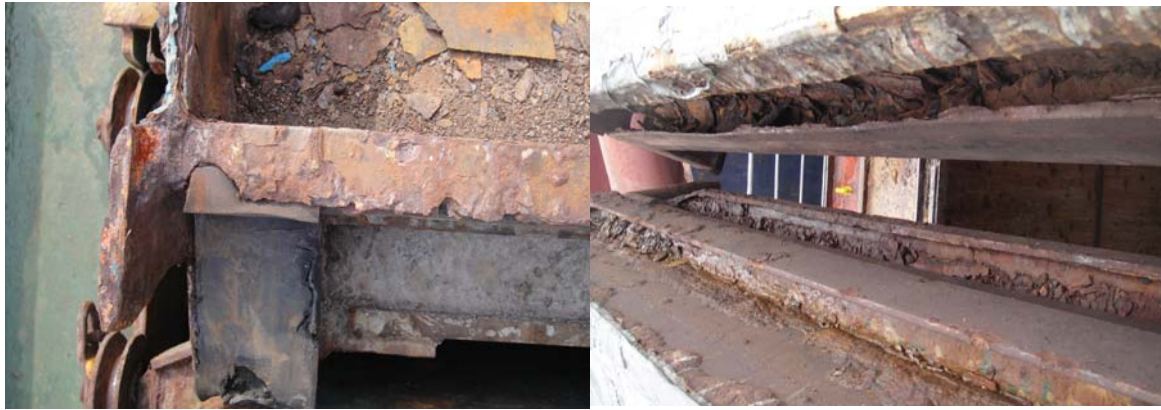
4-2 Seriously corroded rubber channel and draining channel
