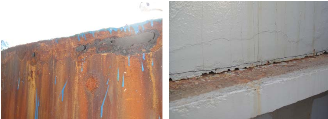
4-3 Seriously corroded skirt plate
