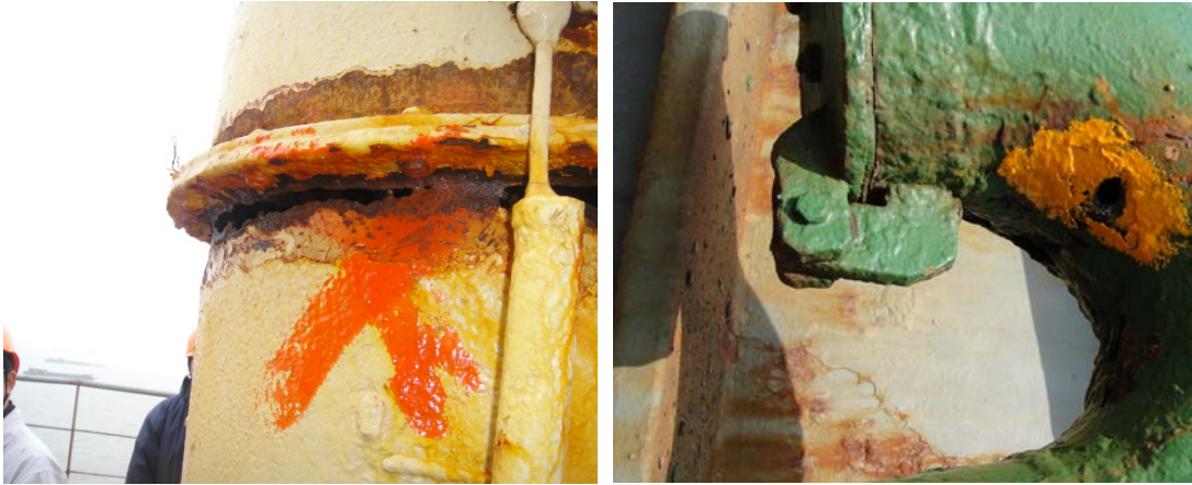
Figure 6 Holed ventilator and air pipe
